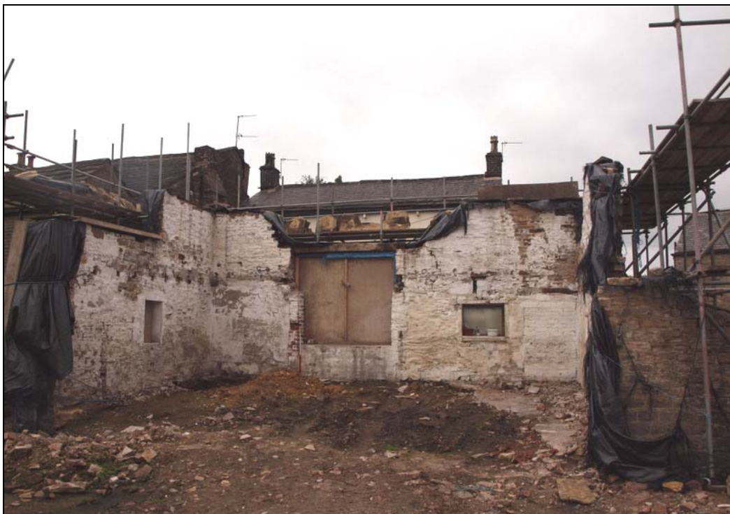
Plate 8: Interior and remains of north-east wall at right of plate
