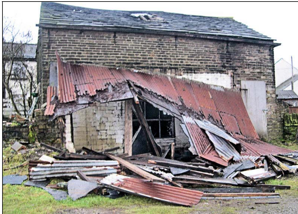
Plate 10: North-east wall after collapse of lean-to, taken 10/1/11. Courtesy of Trevor Jones.
