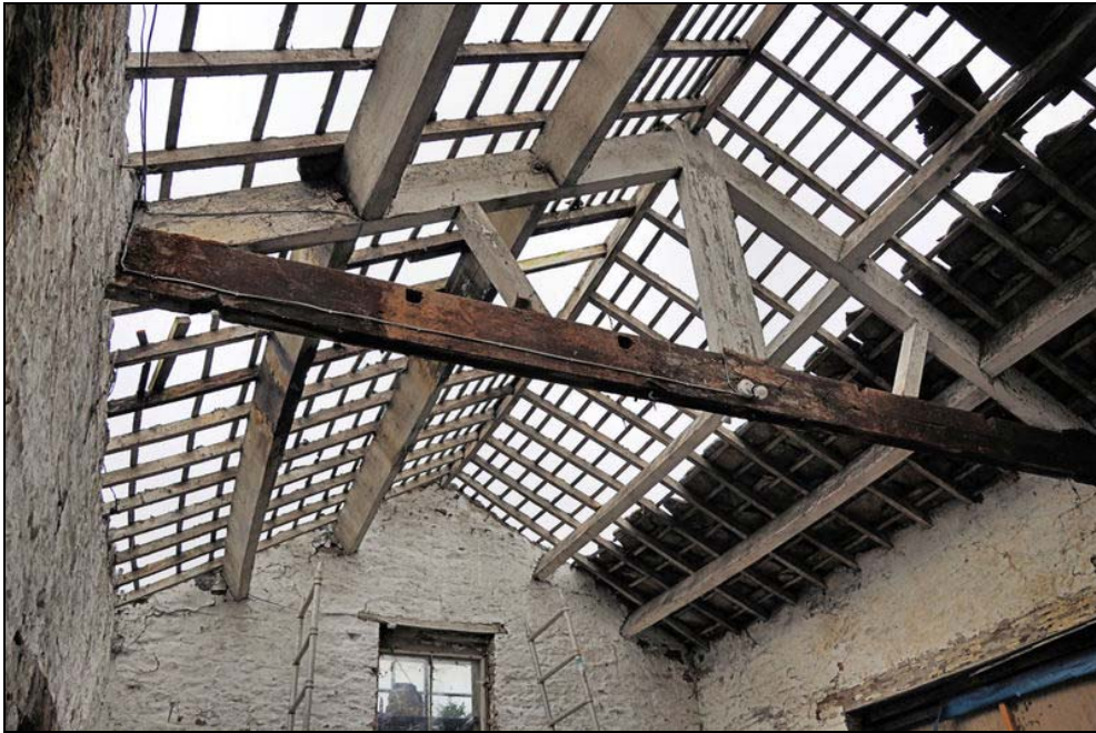
Plate 17: Interior showing king post truss and window in south-eastern gable, taken 21/2/11. Courtesy of Trevor Jones.
