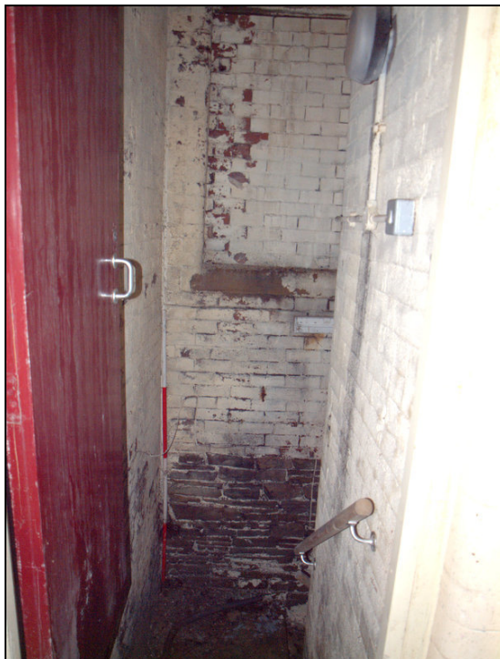
Plate 44: Staircase to basement showing blocked window and changing wall construction
