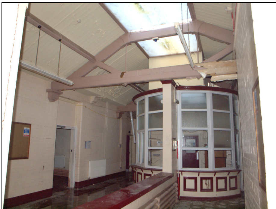
Plate 36: Southern end of central atrium, ground floor, showing the office and truss above
