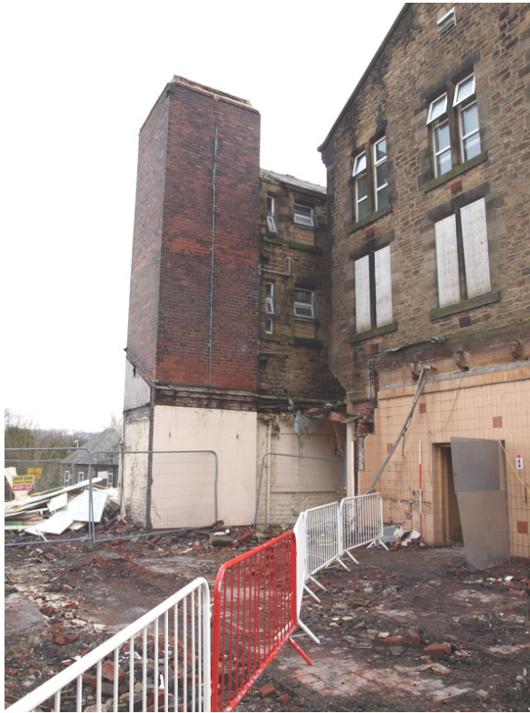
Plate 51: West elevation of central atrium, north end, after removal of north block
