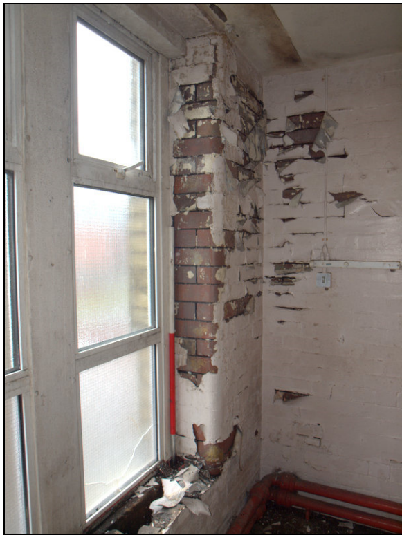
Plate 35: Bare brickwork where paint has peeled away
