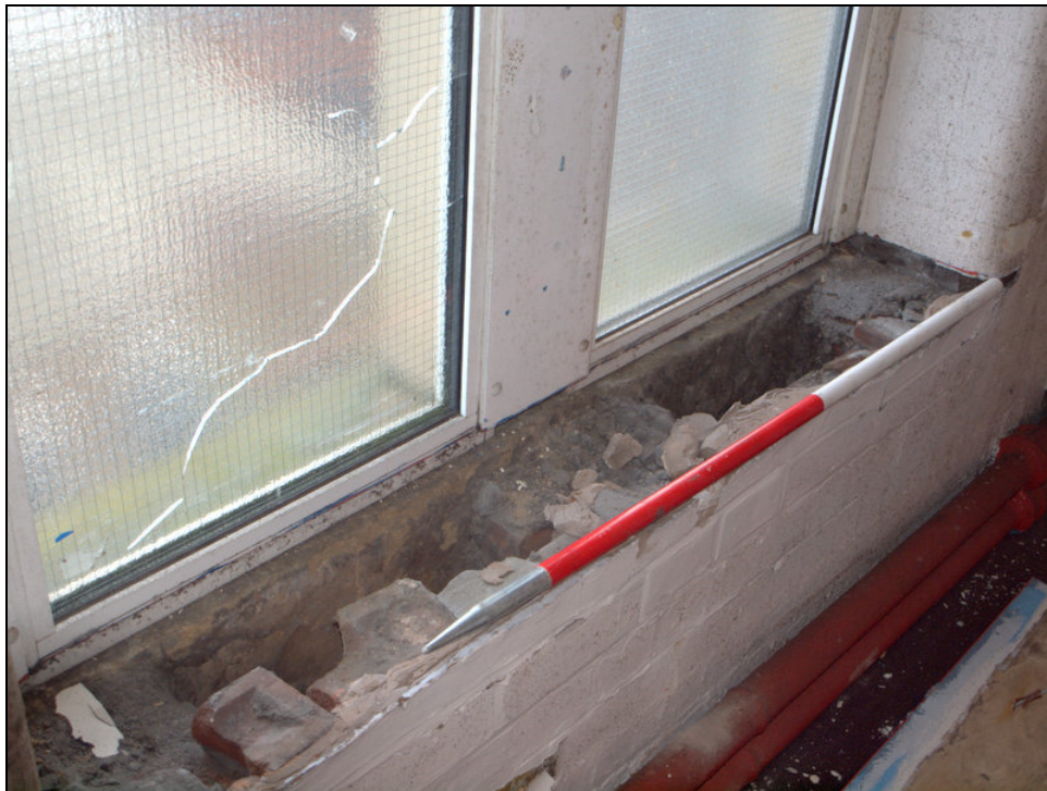
Plate 25: Removed window cill showing brick construction with stone outer skin
