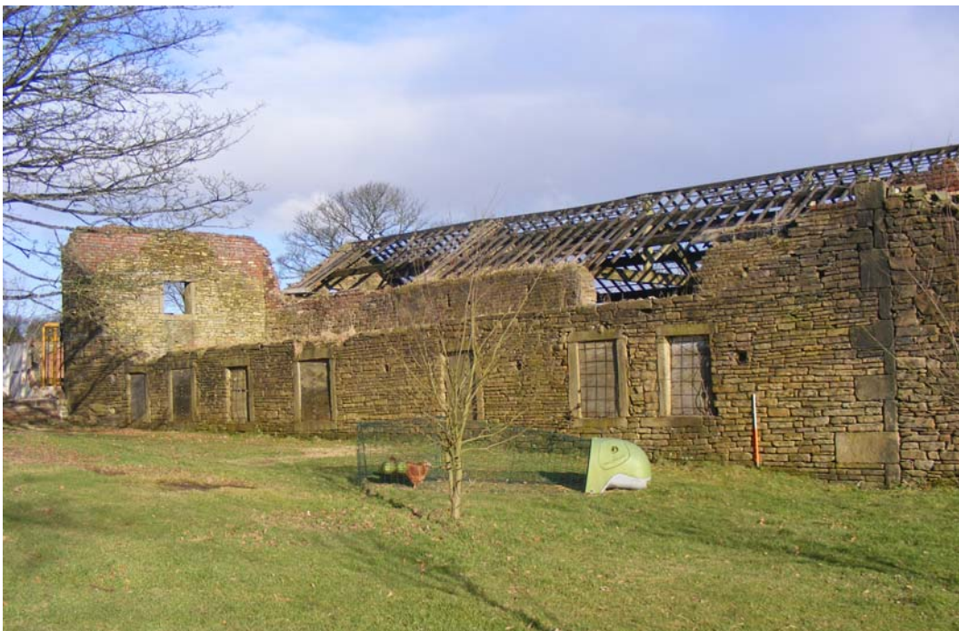
Plate 14. South shippon – south elevation with barn roof beyond
