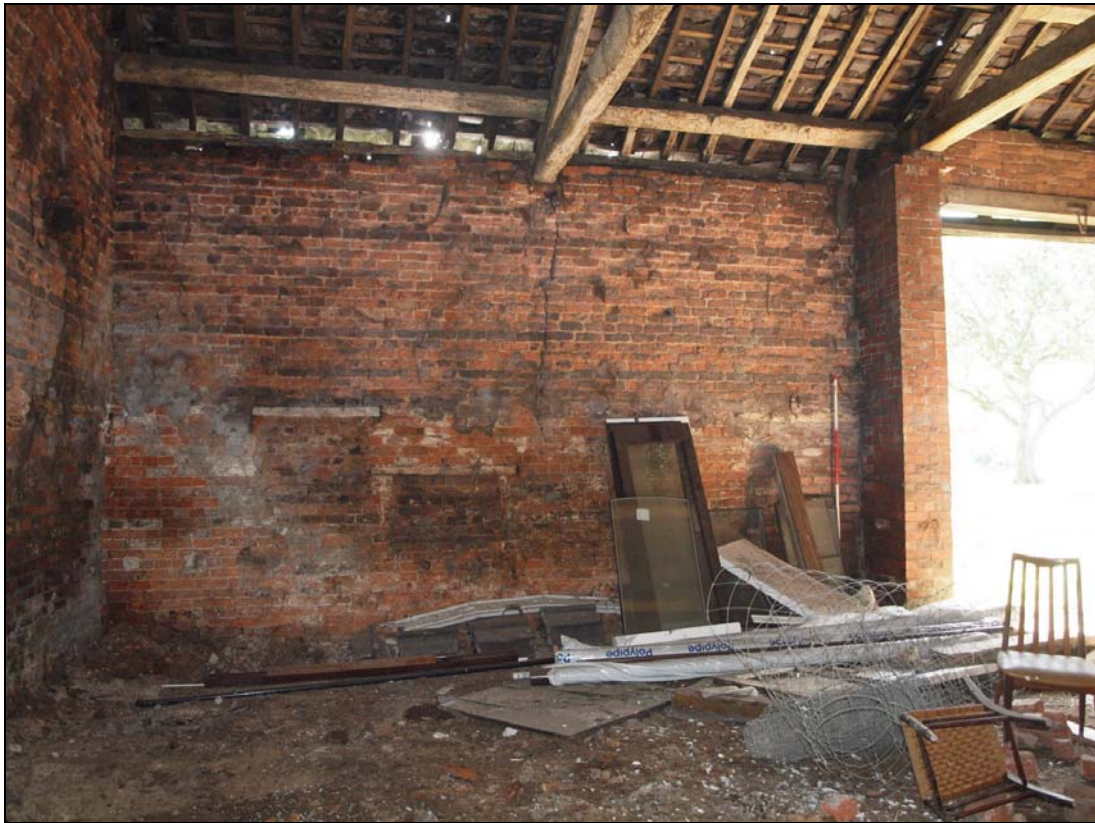
Plate 11: Blocked windows in north end of barn east wall
