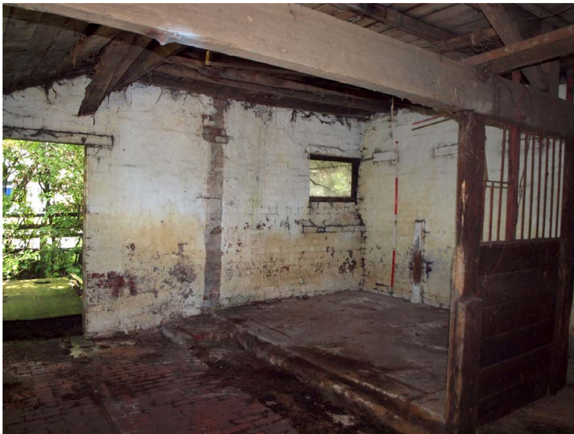
Plate 16: North wall of shippon. Note the brick and concrete areas of the floor
