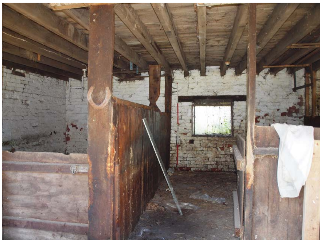
Plate 22: Interior of ground floor of stable; passage between east and central loose box looking south
