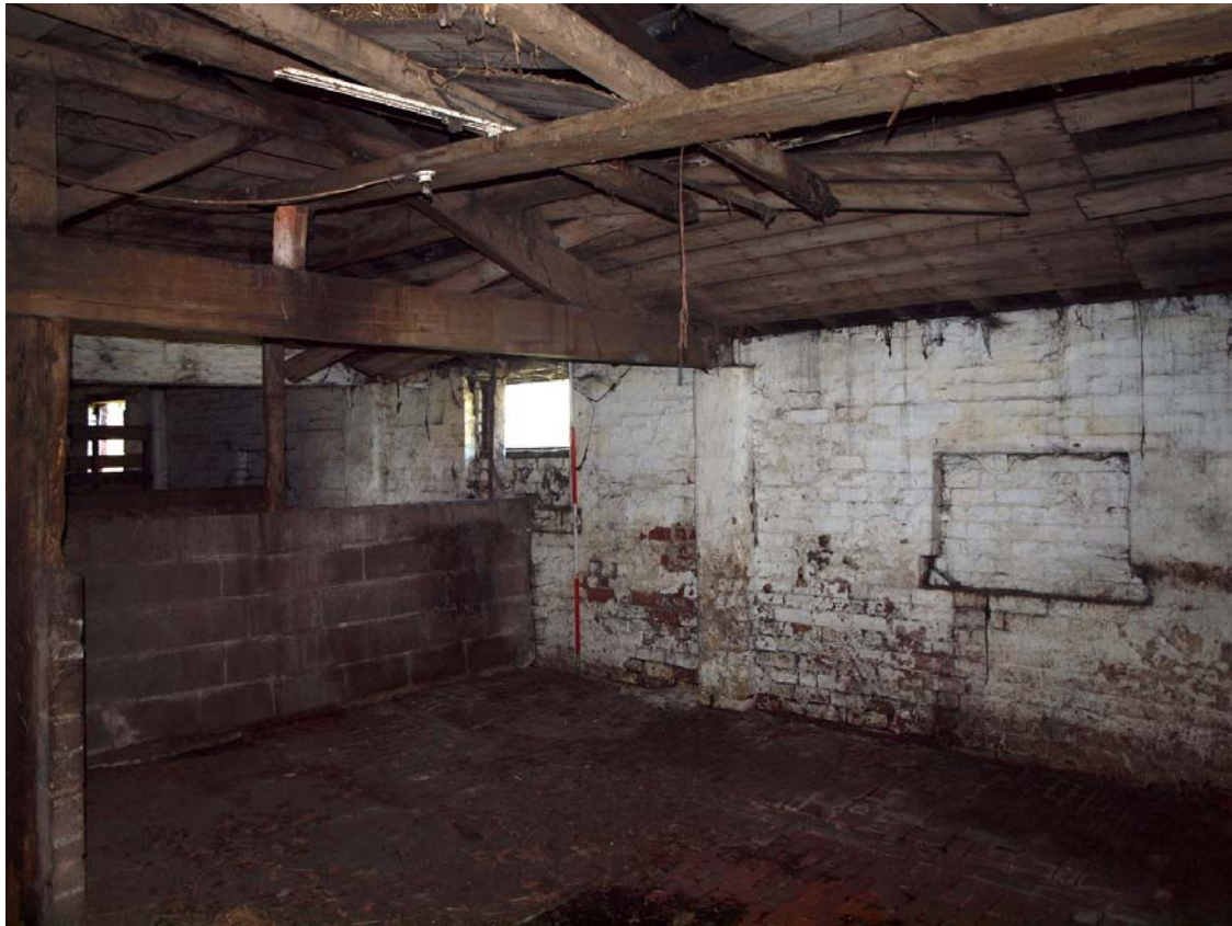
Plate 15: Blocked window in west wall of shippon
