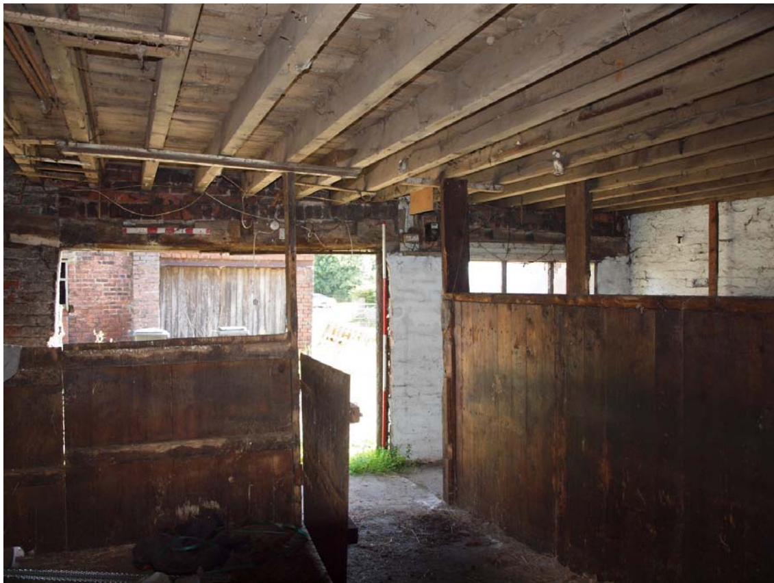
Plate 23: Interior of ground floor of stable; central and east loose boxes looking north
