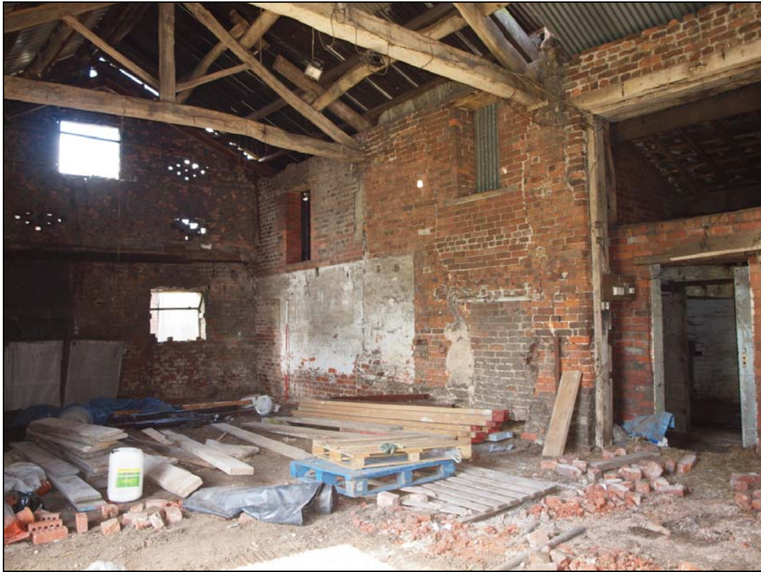
Plate 7: Blocked doorways to the south of barn door.
