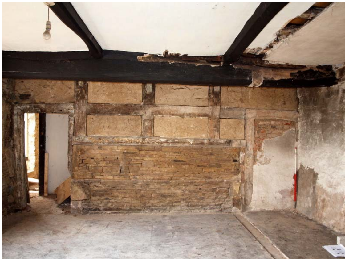
Plate 32: Uncovered timber frame with wattle and daub fill resting on sandstone wall forming west wall of west bay of dwelling
