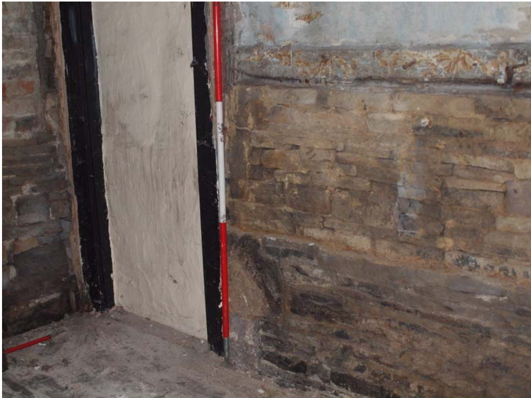
Plate 31: Detail of stone wall and plinth in west wall of west bay of dwelling
