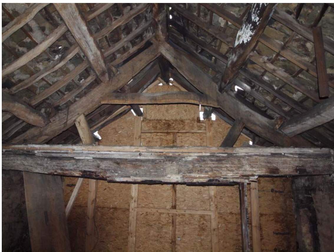
Plate 40: Handcut roof truss at east end of first floor of west bay in central dwelling
