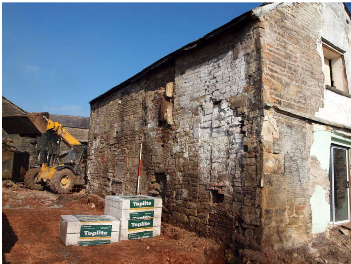
Plate 11: West elevation of wing after removal of western extension. NB blocked windows to left of ranging rod and back of fireplace to right.
