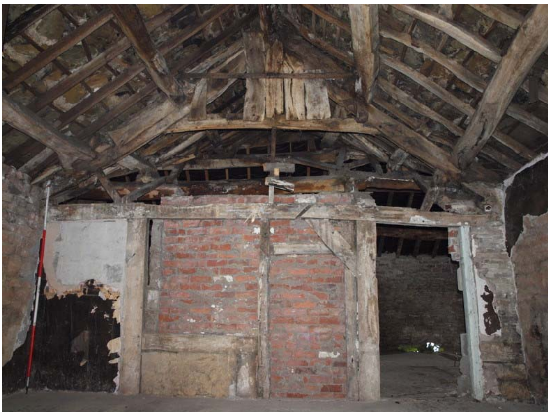
Plate 37: Timber frame in west wall of first floor of central dwelling with handcut roof timbers above
