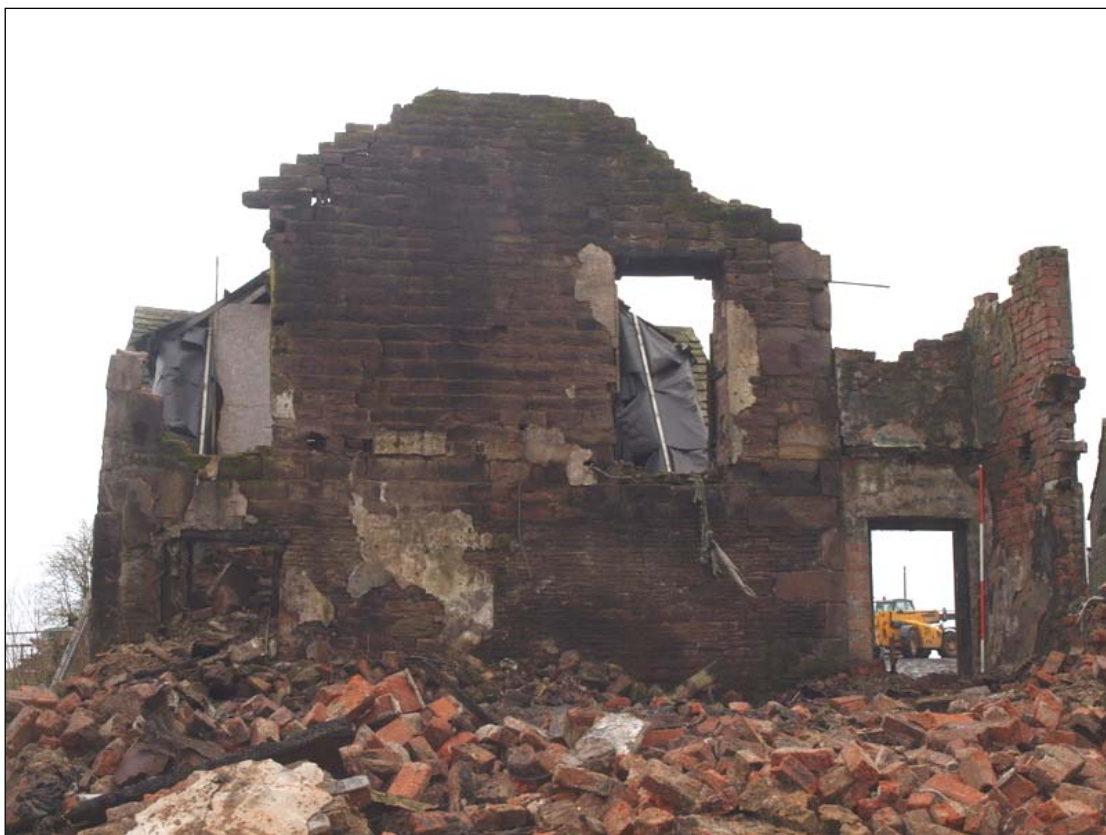
Plate 8: East wall of dwelling after demolition of eastern extension. The right-angled walls and doorway at the right-hand end were part of the extension
