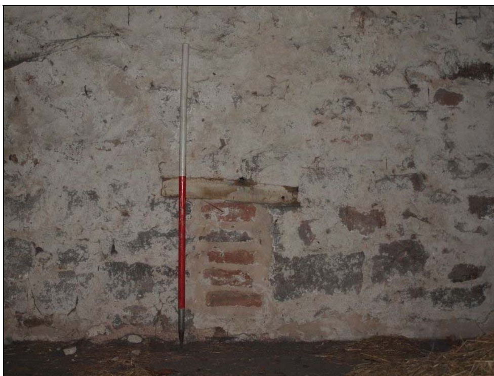
Plate 26: Blocked vent hole in south wall
