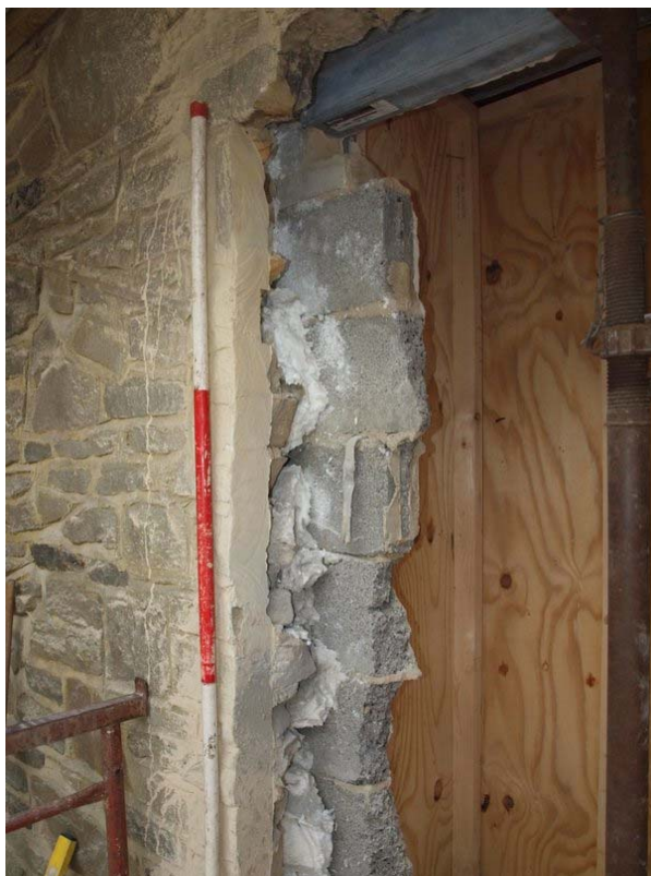
Plate 9/13: Detail of above showing single skin stone with concrete block and insulation
