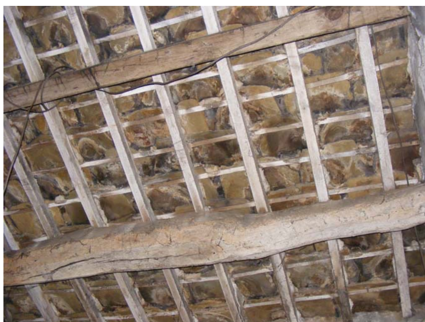
Plate 12: Handcut purlin in south pitch of cottage roof
