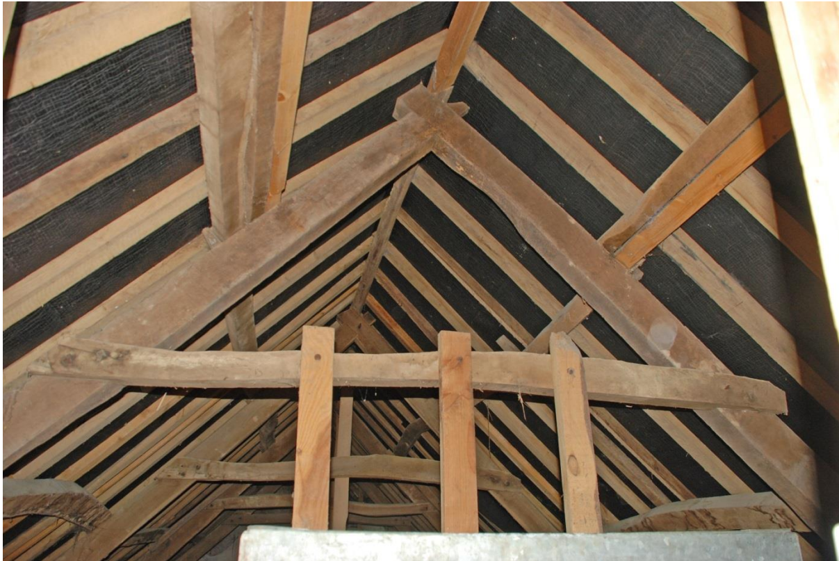
Fig. 16 The 18th-century roof, showing crude construction not intended to be exposed and viewed.
