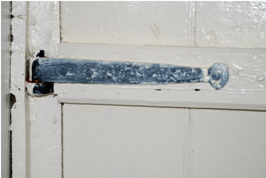
Fig. 5 Strap hinge hung from a pintle on inside of door into central service room.
