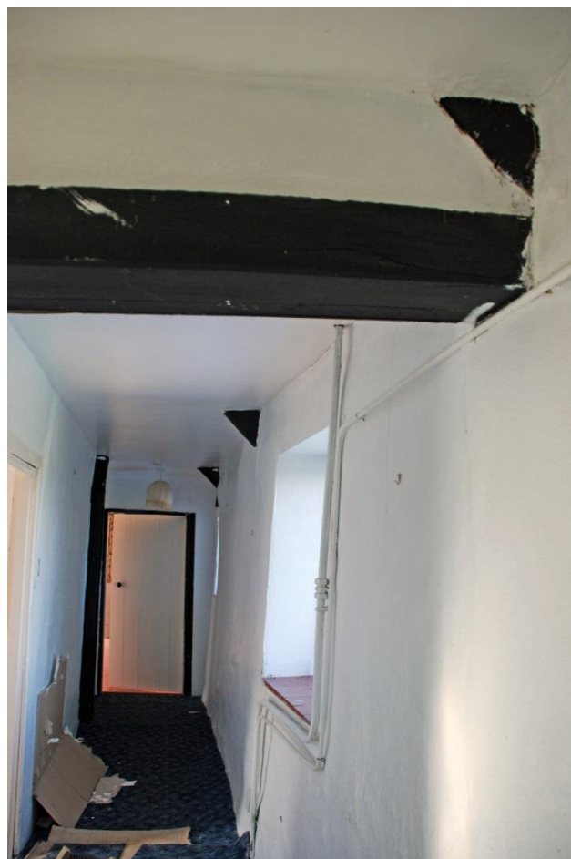
Fig. 18 The north end of the surviving tie/ceiling beam, looking west, showing the ends of two further trusses now without the original tie/ceiling beams beneath them.
