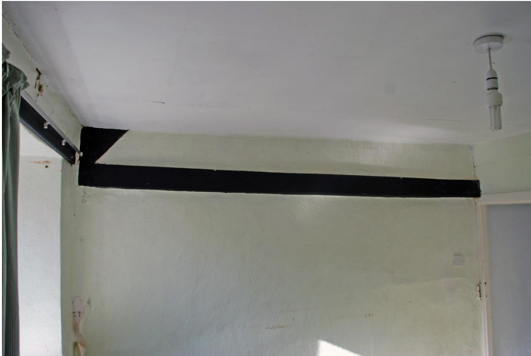
Fig. 17 The sole surviving intact tie/ceiling beam beneath the easternmost truss, looking west.
