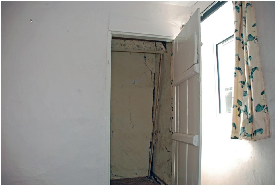
Fig. 12 The cupboard in the master bedroom, showing a surviving section of tie/ceiling beam.
