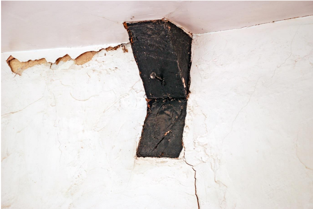
Fig. 19 The sawn-off stub of the tie/ceiling beam beneath the westernmost truss in the master bedroom.
