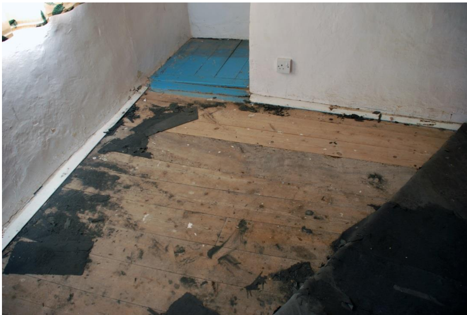
Fig. 13 A wide oak floor board (toward the rear) survives in the master bedroom amongst later narrower replacements.
