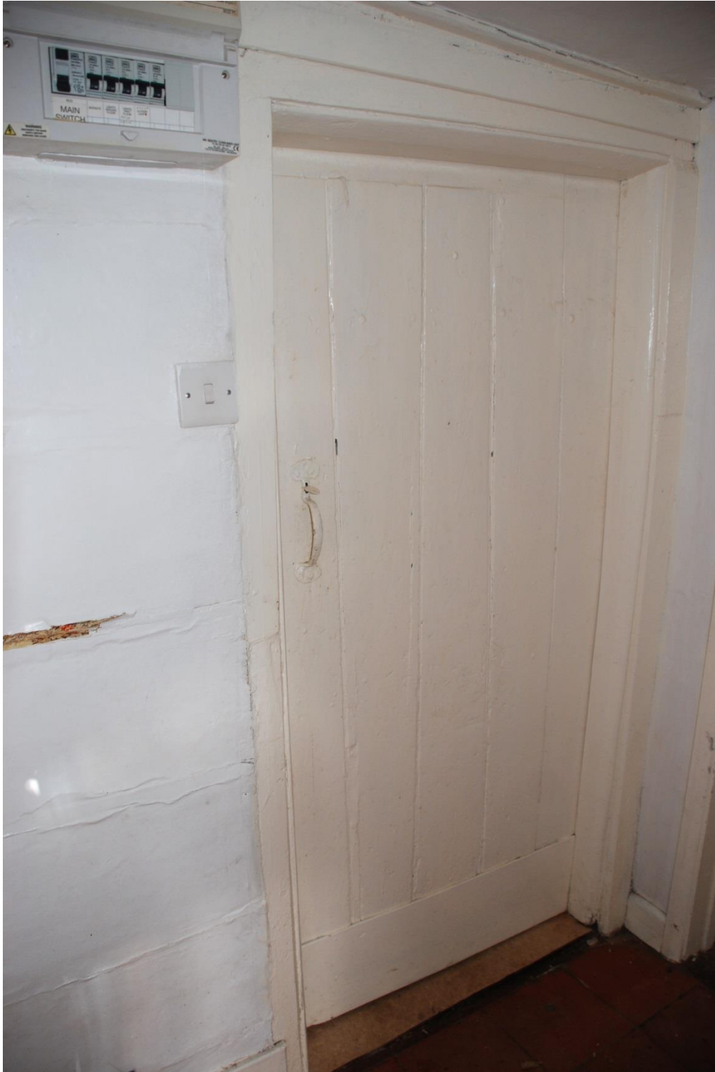
Fig. 3 The horizontal planked side wall of the lobby and plank and batten door leading into the central service room.
