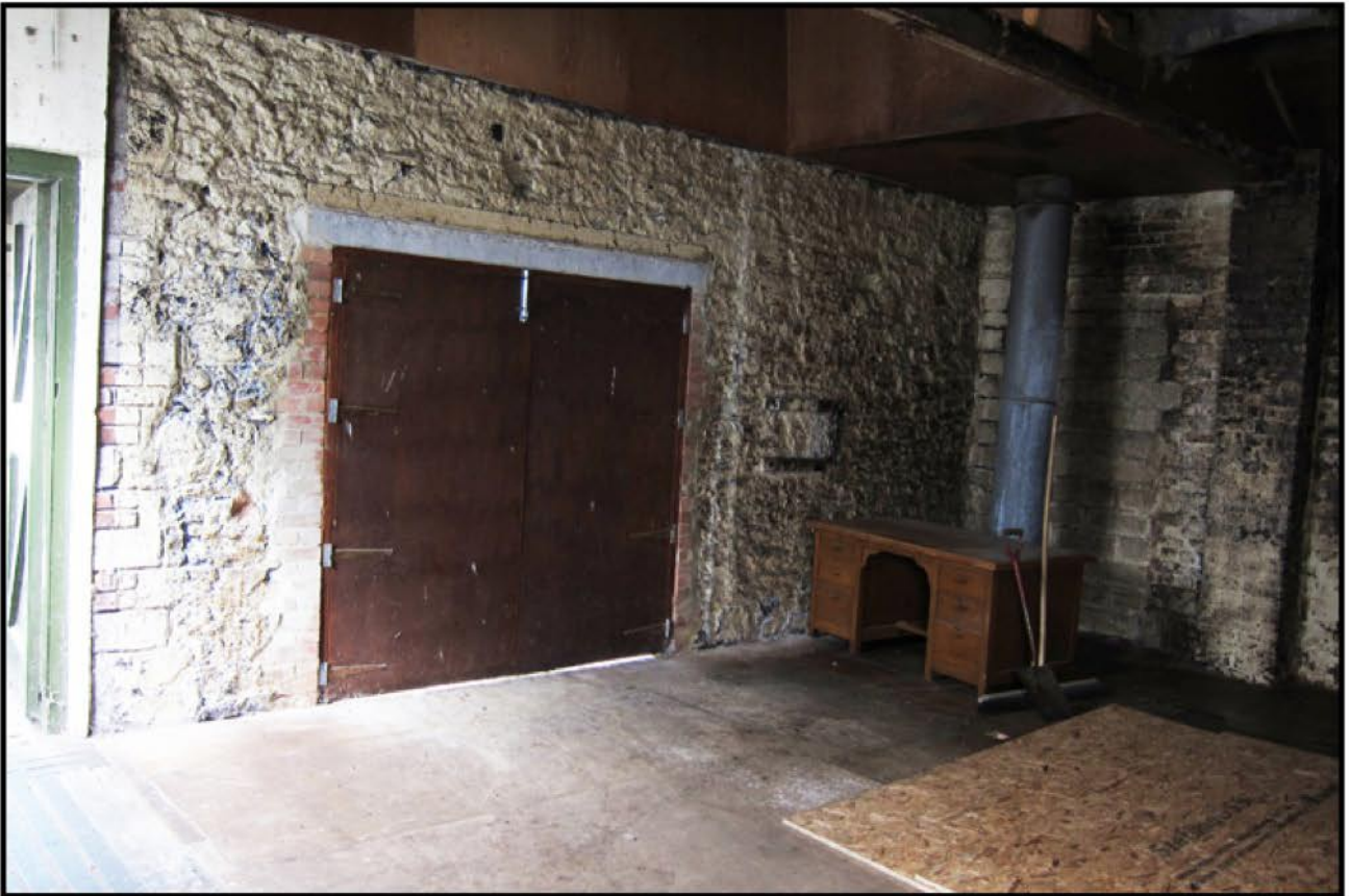
Photo. 13 The western interior to the partial nineteenth-century range within Building J, showing the surviving end wall, the side wall shared with the range to the north, and the end to an original roof truss, resting on this wall.
