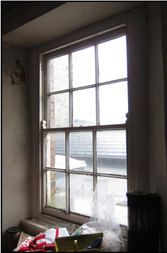
Photo. 5 A sash window on the north side of first floor to Building B.
