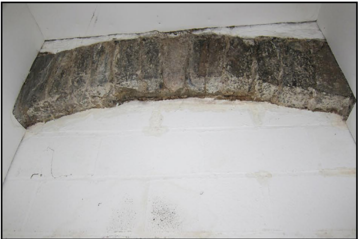
Photo. 6 The blocked entrance at the west end of the ground floor to Building B.
