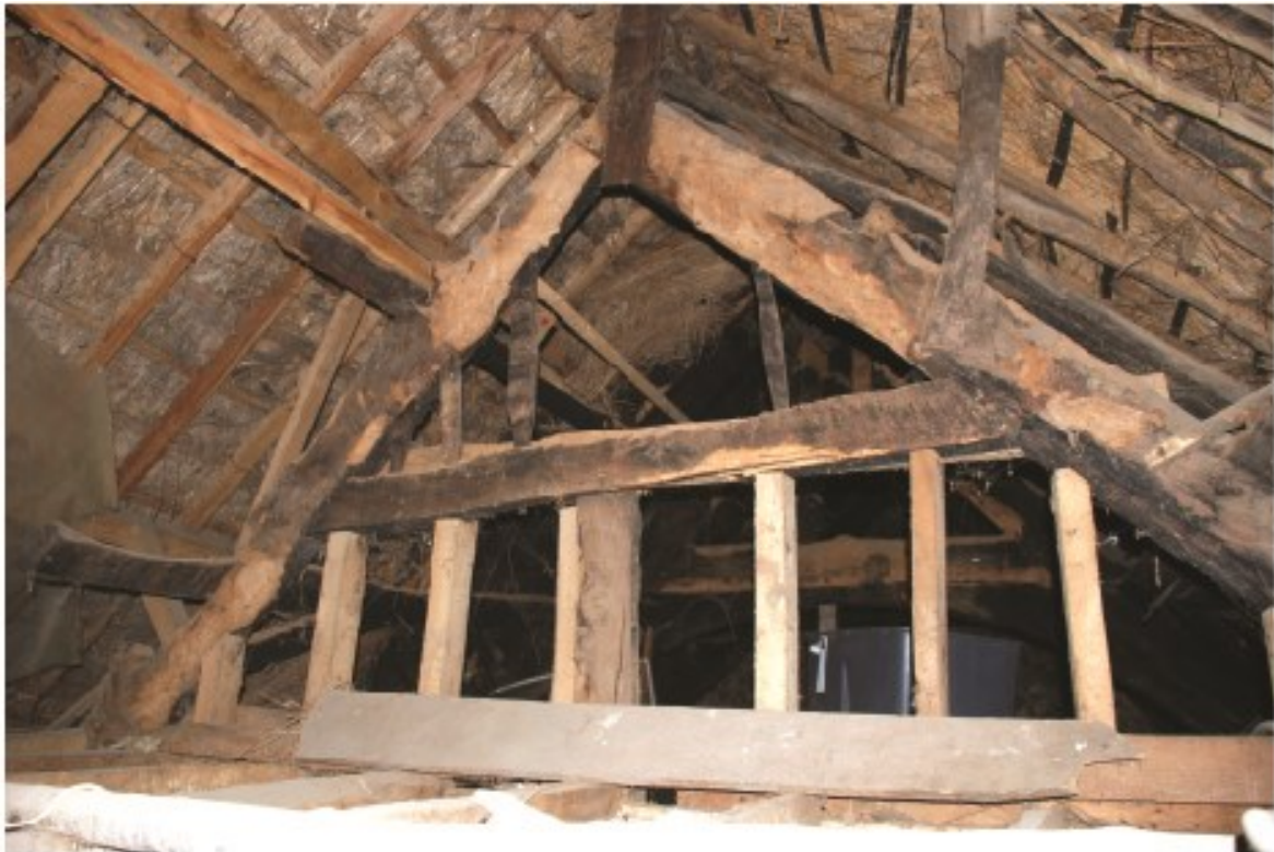
Plate 17 The early 17th-century A-frame truss supporting the east end of the medieval roof, showing struts nailed to its east side to support the phase 2 purlins and ridge, looking west.
