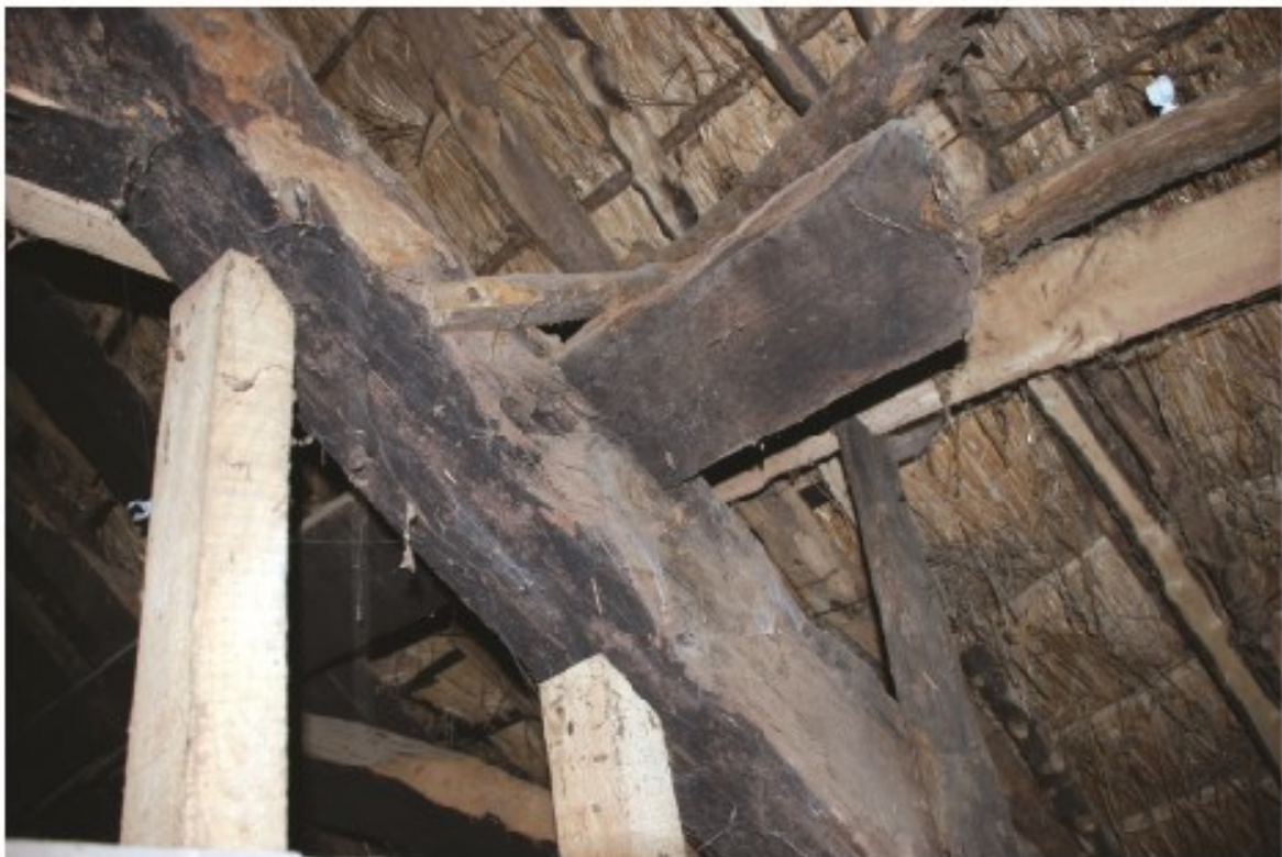
Plate 18 Close-up showing east end of medieval purlin supported by early 17th-century A-frame truss, and strut with v-shaped notch at its top supporting lower purlin of the later roof, looking northwest.
