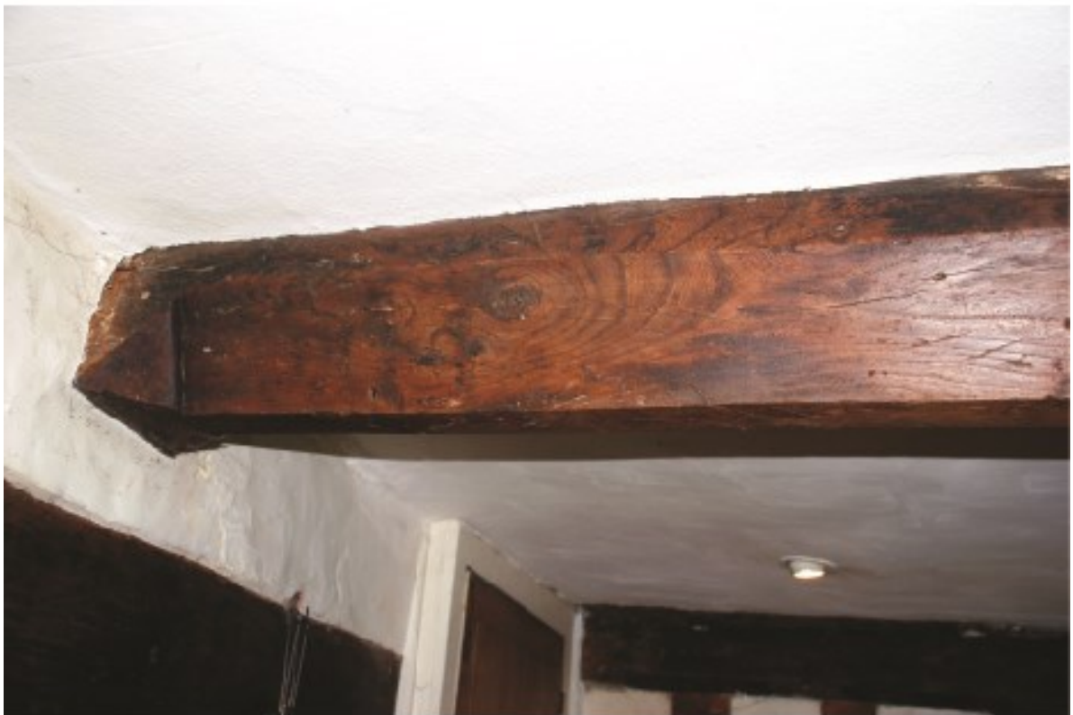
Plate 24 Phase 4 floor beam inserted into the formerly open hall, showing deep chamfer and stepped stop, looking northeast.
