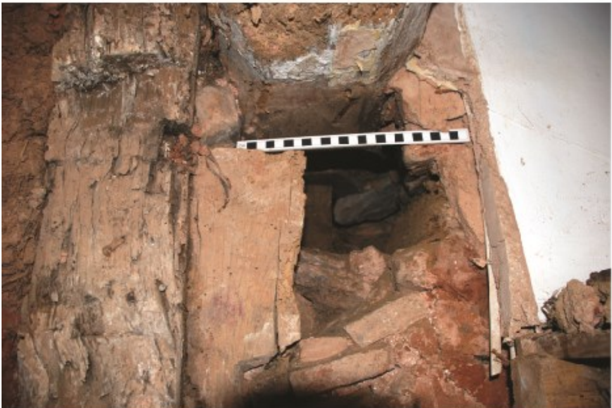
Plate 30 Rubble and brick packing beneath the 19th-century first-floor beam to the east of the cross-passage, and showing damage to the former wooden window in the south wall, looking south
