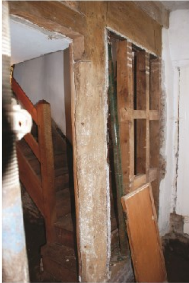
Plate 21 The kitchen and stair doorways through the screen on the lower side of the passage, showing the higher door head of the stair doorway, looking southeast.
