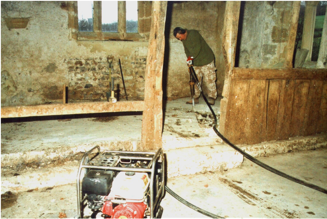
Plate 1 Removal of modern concrete, showing spin in the floor at the medieval screen.
