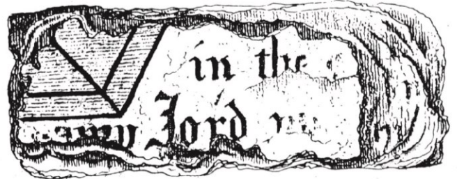
Successive coats of plaster coloured and inscribed, found under the whitewash over the old Chancel arch in the nave. — since gone to pieces.
