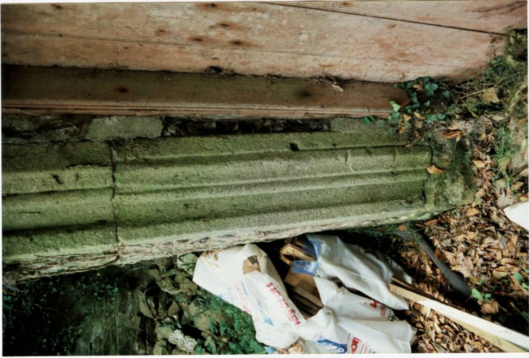
Plate 26. Detail of granite door surround showing jamb stone re-used from a window.
