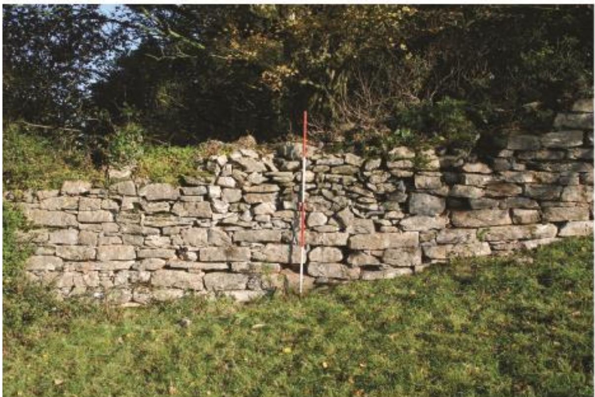
Plate 22 The wall in North Tor showing small post-medieval or modern repair, looking northeast.
