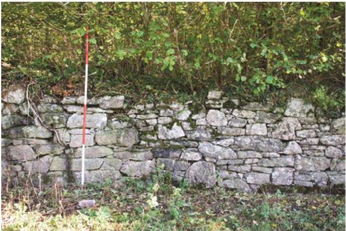
Plate 20 The wall in Custer Park showing change in character of construction, looking east.
