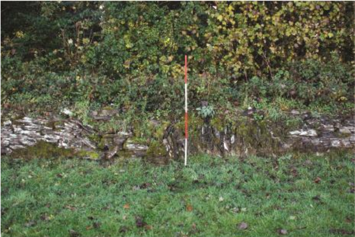
Plate 23 The wall in Yonder Kit Hill showing post-medieval repair using pitched stones, looking southeast.
