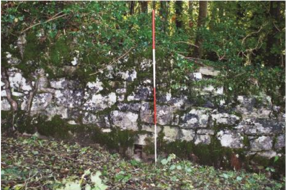
Plate 19 The wall in Custer Park showing random rubble construction and hole low down, looking south.
