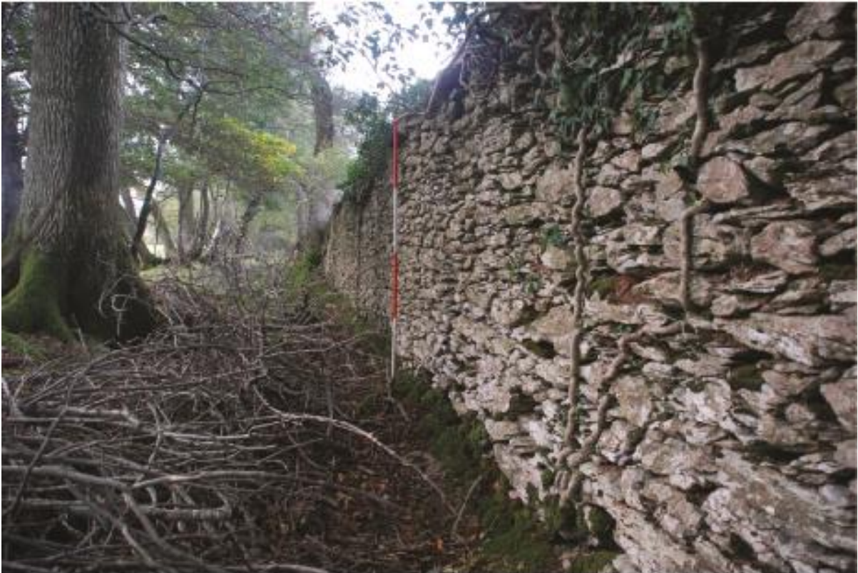
Plate 15 The wall in Bird showing striated weathering pattern on stones, looking northwest.
