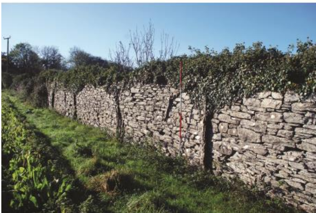
Plate 8 A well-preserved section of wall between North Tor and Bird which once separated off a close within the deer park, looking southwest.
