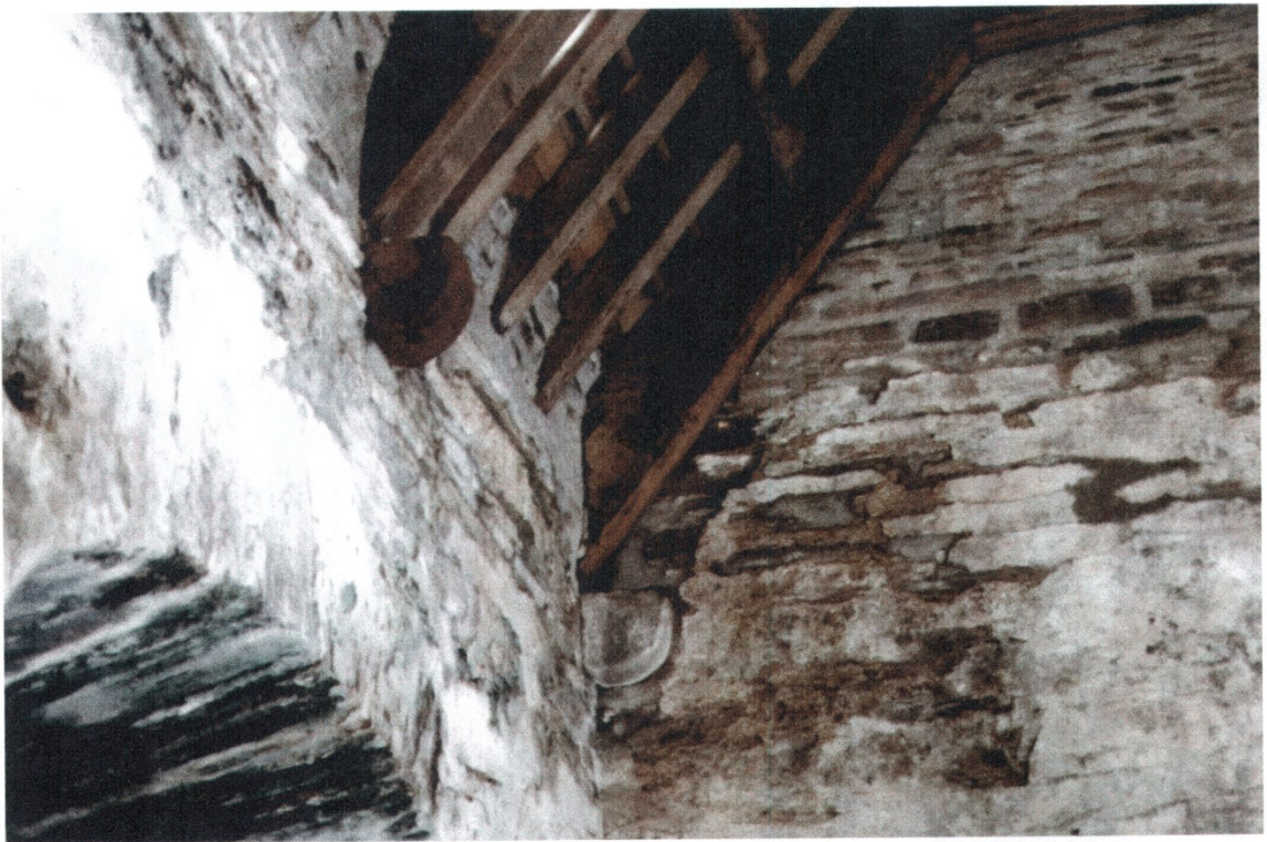
Plate 2 The west wall of the chapel showing a scar above the corbel for an arched brace.
