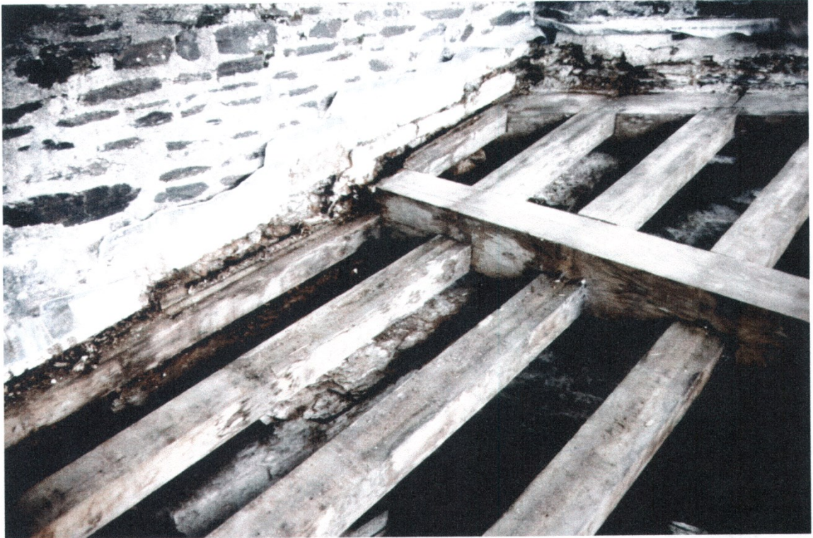
Plate 1 The roof joists of the western tower showing rot.
