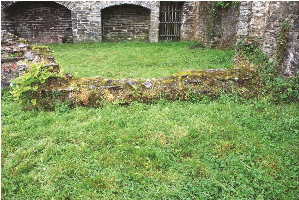
Plate 22 The north terrace and former kitchen area before construction of new access ramp, looking southeast.
