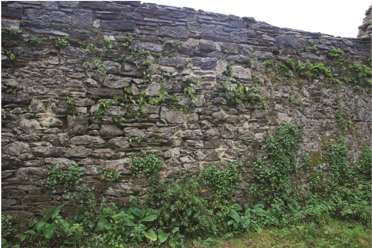
Plate 25 The boundary wall before re-pointing, looking east.
