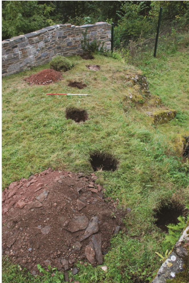
Plate 20 Excavation of post-holes for new rail across the north terrace, looking north.
