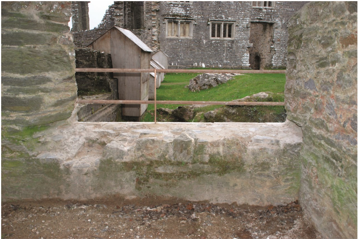
Plate 13 The kitchen quarter after conservation work, new railing and consolidation of the window sill, looking northeast.
