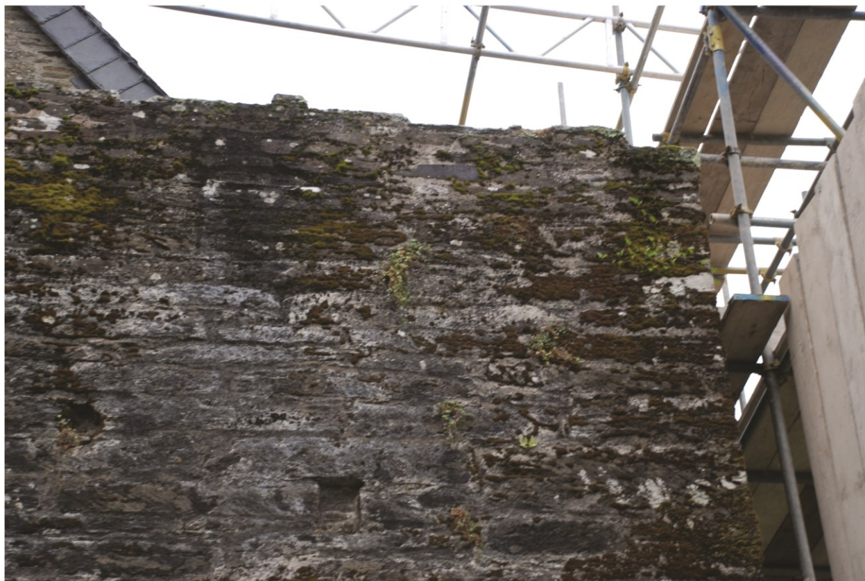
Plate 4 The gatehouse parapet wall, NE corner, before conservation work, looking southwest.
