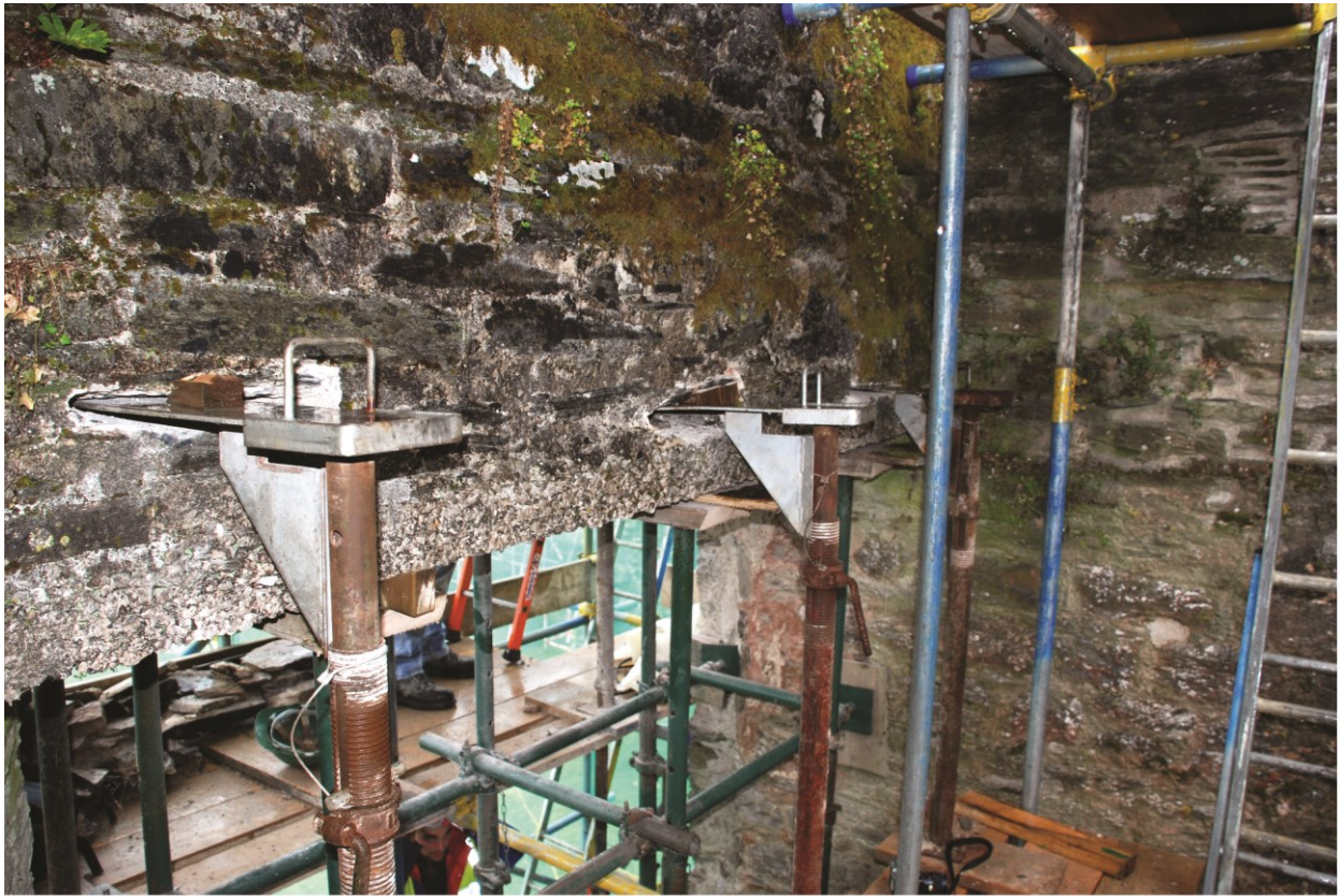
Plate 7 The kitchen quarter, first-floor concrete lintel before conservation work, looking east.
