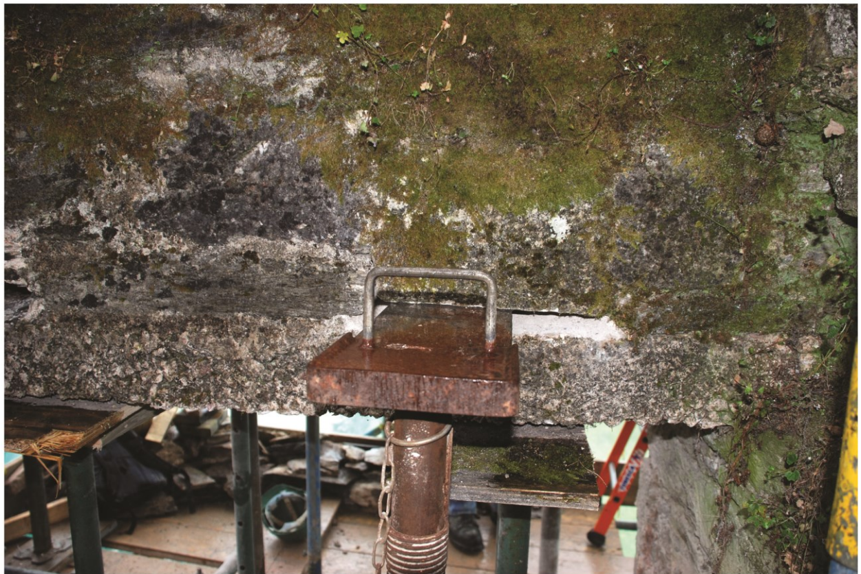
Plate 8 The kitchen quarter, first-floor concrete lintel before conservation work, looking northeast.
