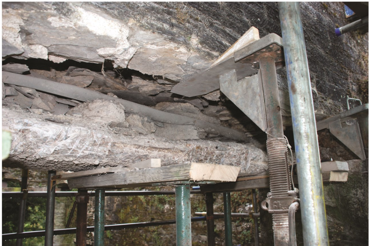
Plate 10 The kitchen quarter, second-floor concrete lintel before conservation work, showing previously inserted tie, looking west.
