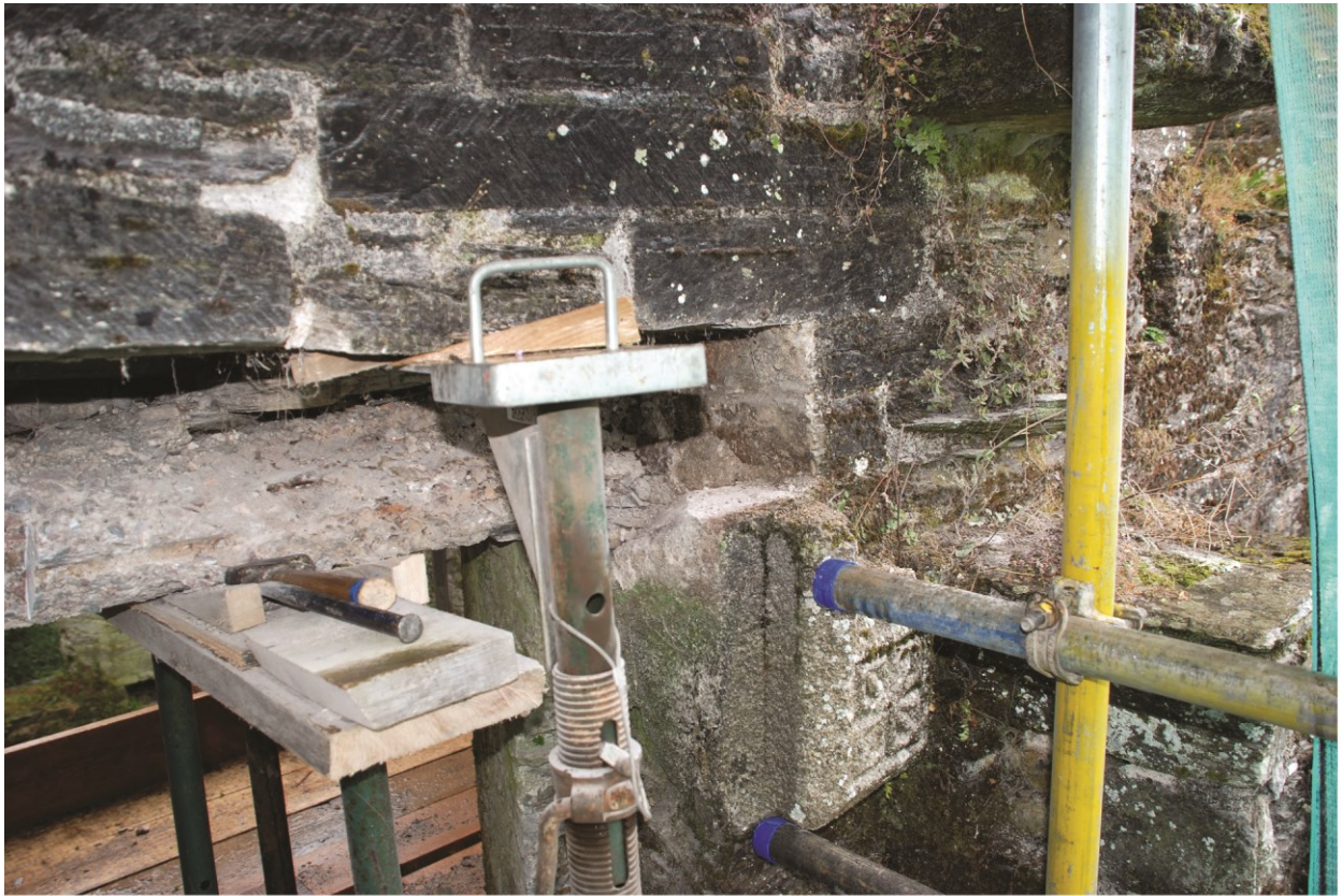
Plate 9 The kitchen quarter, first-floor concrete lintel before conservation work, looking west.
