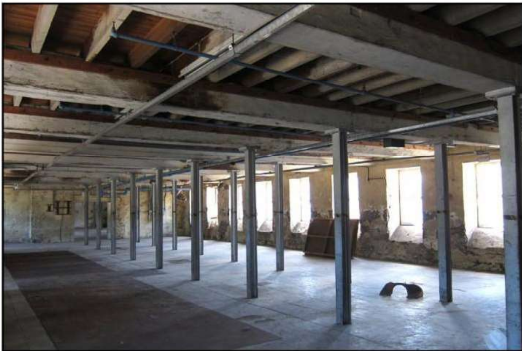
Photo. 10 North range first floor, showing window and second-storey floor details, looking southwest.
