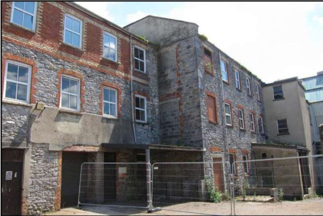
Photo. 17 Junction between the north and south ranges on the west side, showing the blocked entrances on the south range north elevation, looking SSE.
