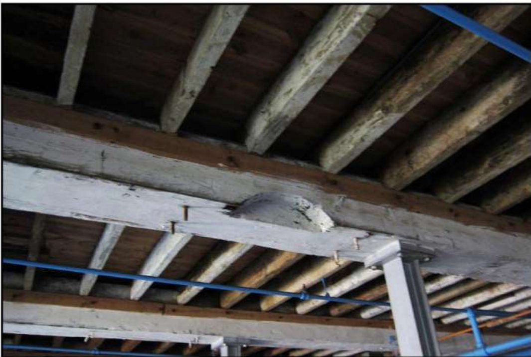
Photo. 18 The power transmission retaining bolts and cutout floor bearer in the basement of the south range, looking SSW.
