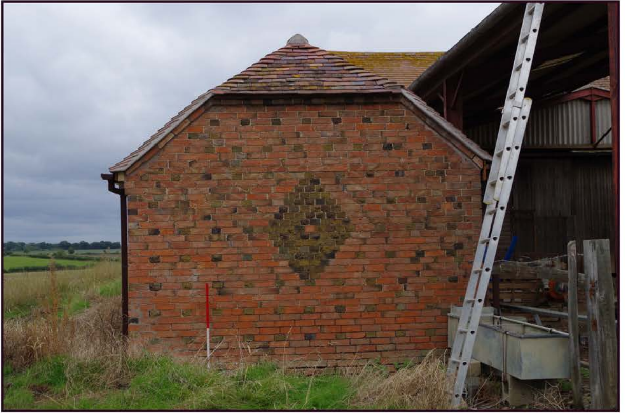
Fig 16: Phase 2 shelter shed/implement shed; south elevation showing diaper work in over-fired bricks
