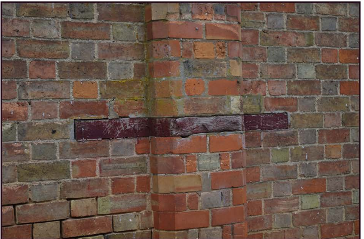
Fig 10: Phase 3 cart shed and stable; east elevation, detail of timber inserted in buttress
