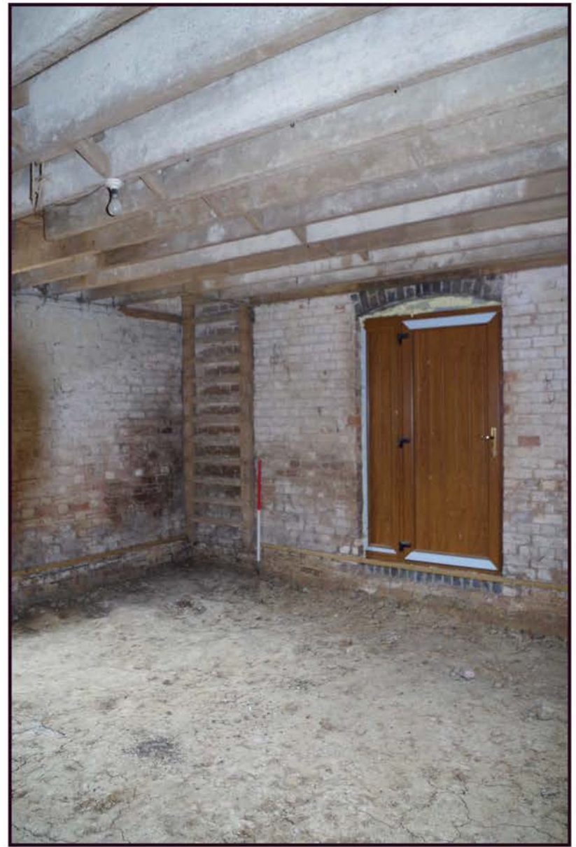
Fig 20: Phase 3 cart shed and stable; ground floor, showing ladder to hay loft
