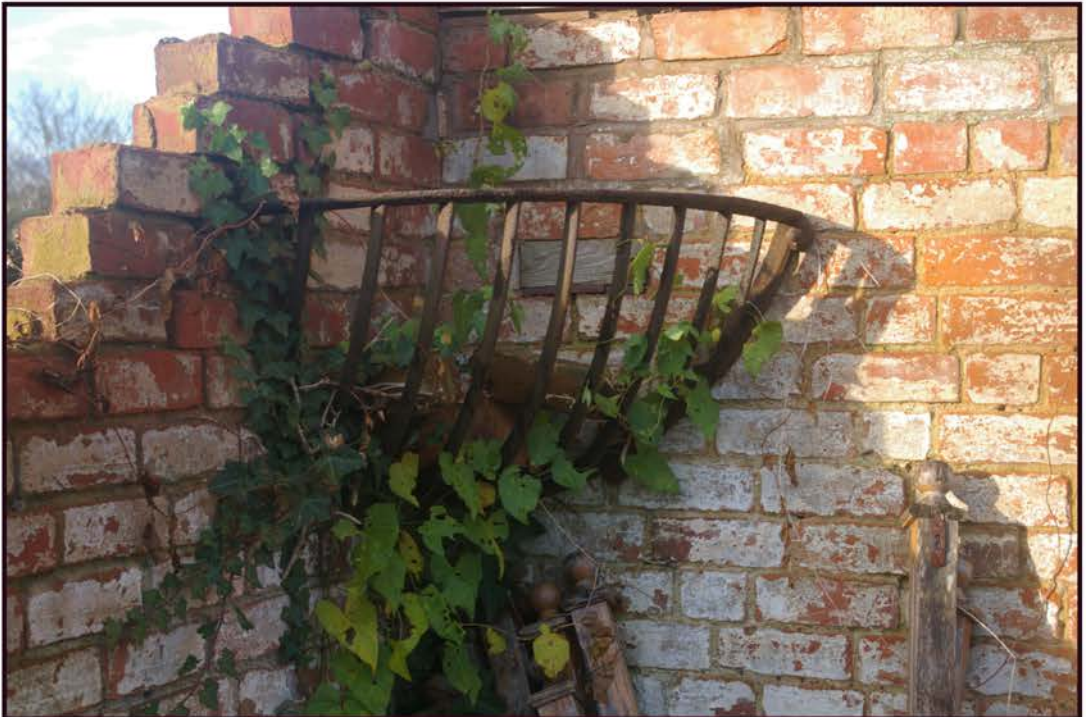
Fig 18: Feeding basket in collapsed part of stable
