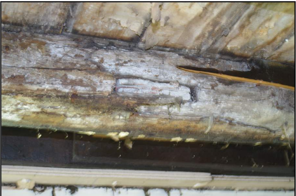
Fig 9: Phase 1, ground floor; showing re-used ceiling joist with redundant mortice and tenon joint
