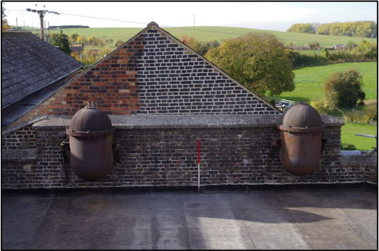
Fig 7: General view of both mufflers from east
