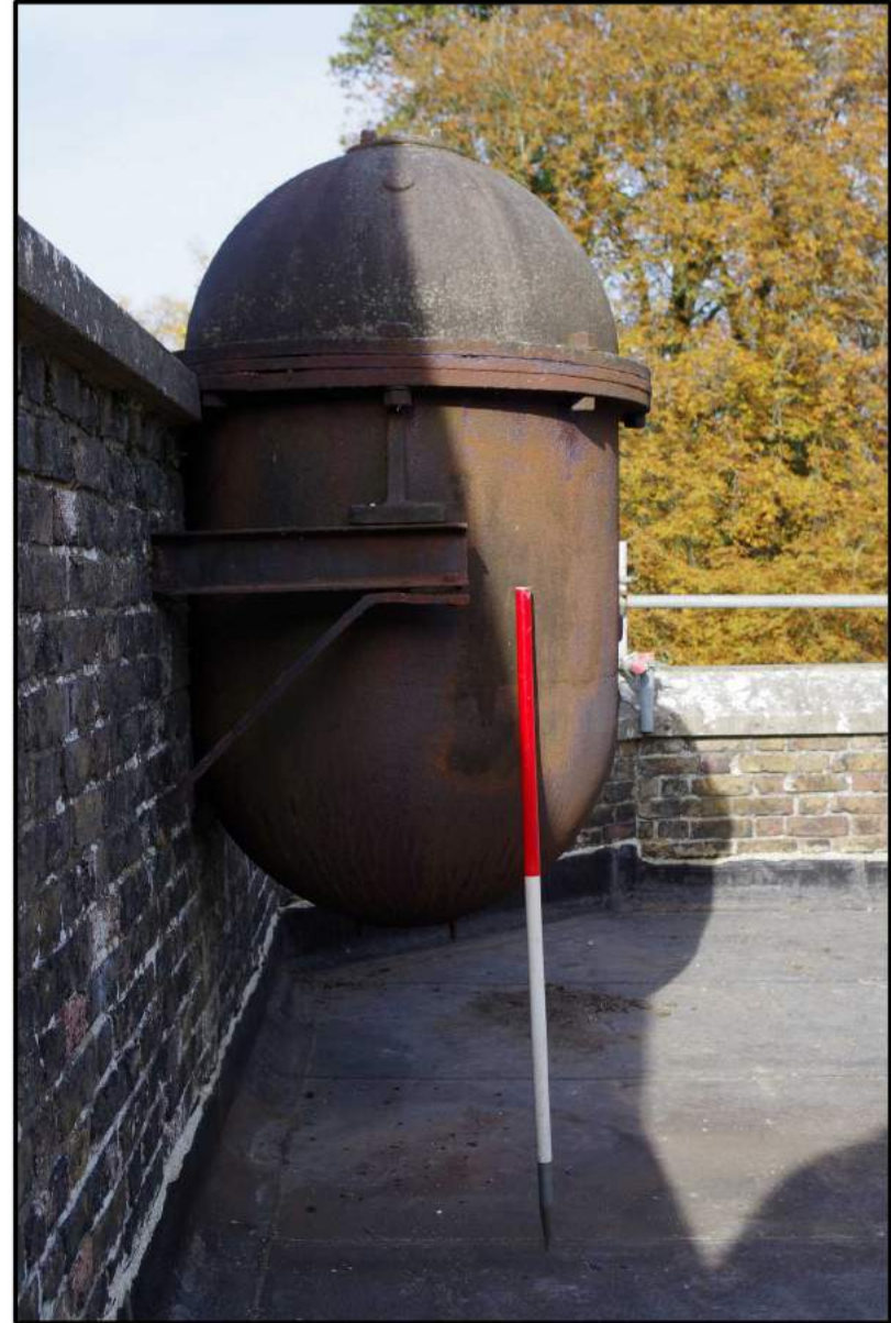
Fig 4: Northern muffler; view from south
