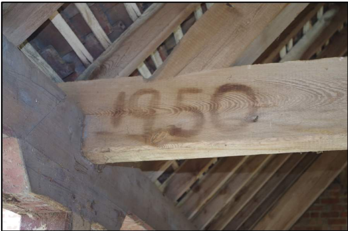
Fig 23: North end, showing graffiti on tie beam
