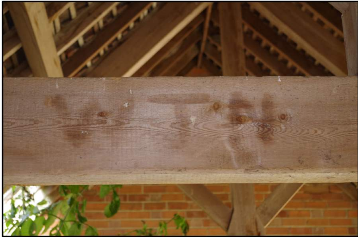
Fig 24: North end, showing graffiti on tie beam
