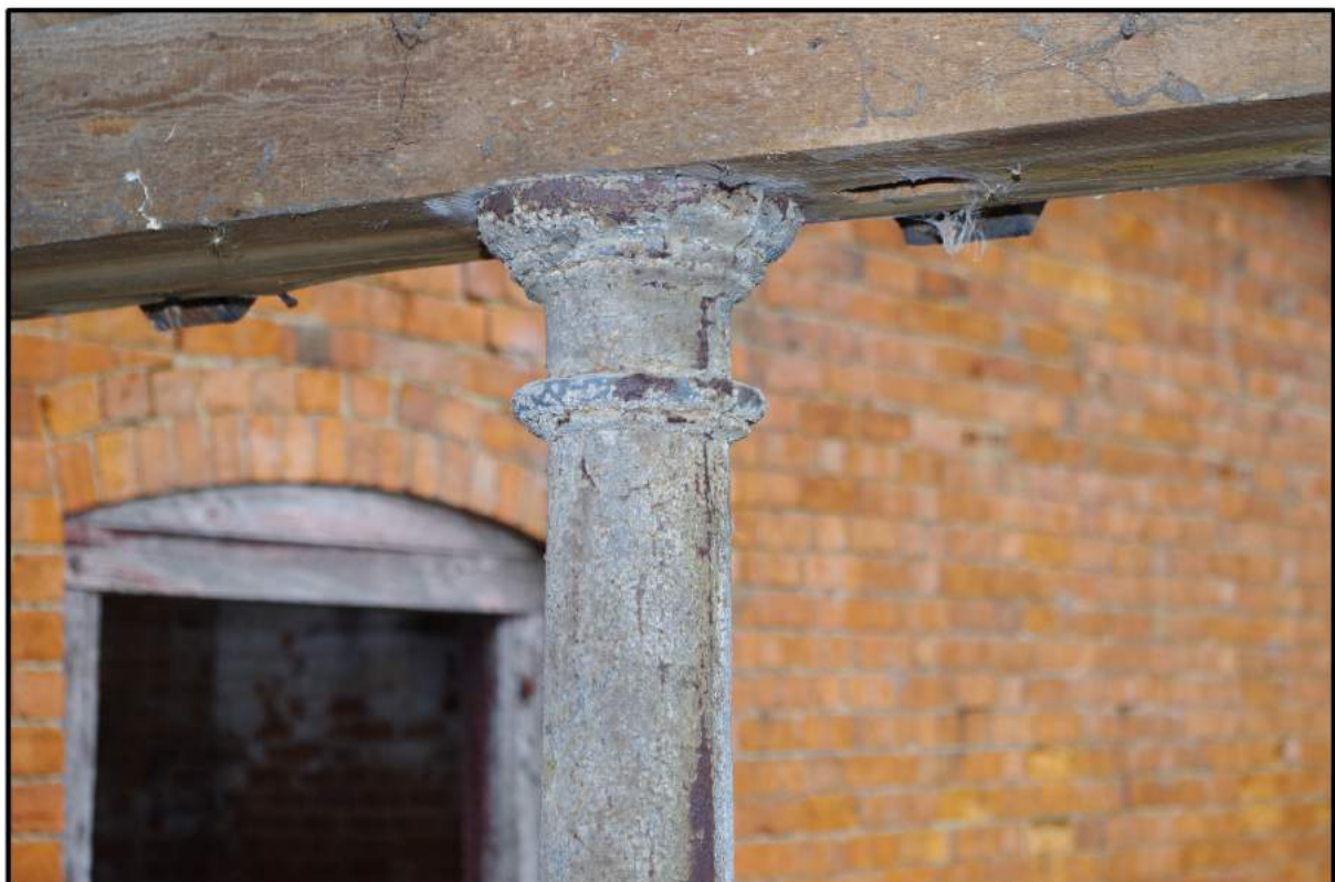
Fig 31: Southern end, detail of cast iron column
