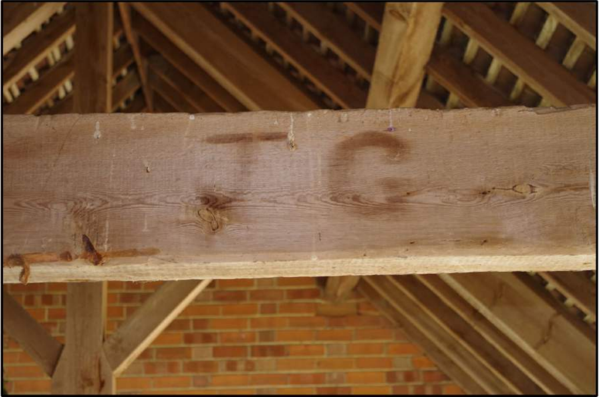
Fig 25: North end, showing graffiti on tie beam
