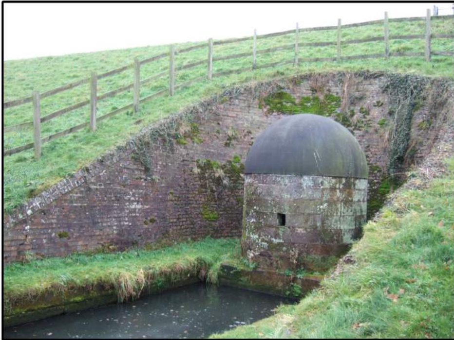
Fig 11.5: Valve house at Belvide reservoir, Shropshire Union Canal
