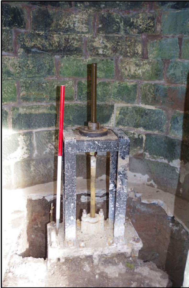
Fig 8: View of the valve support
