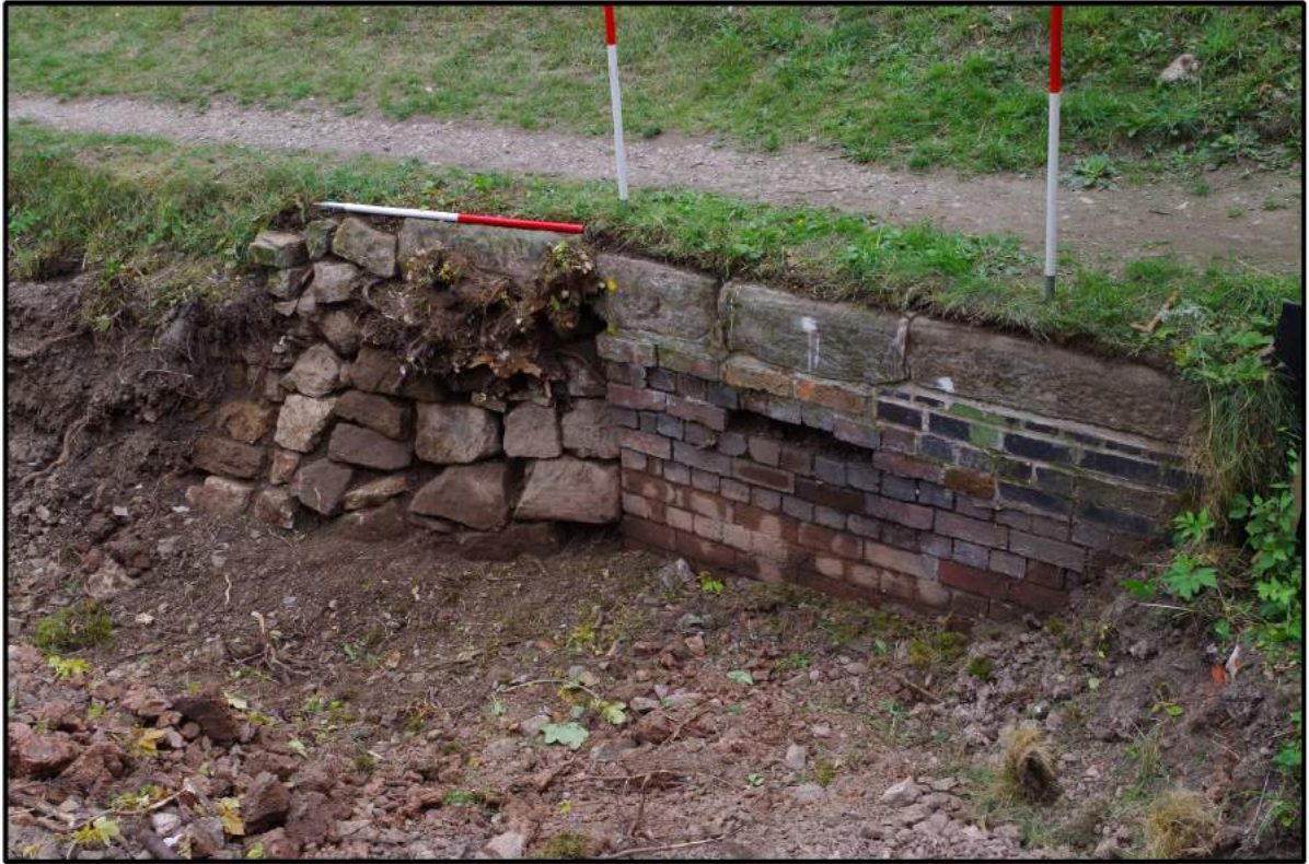
Fig 6: View of the nearside towpath stone rubble retaining wall, Montgomery Canal, Crickheath
