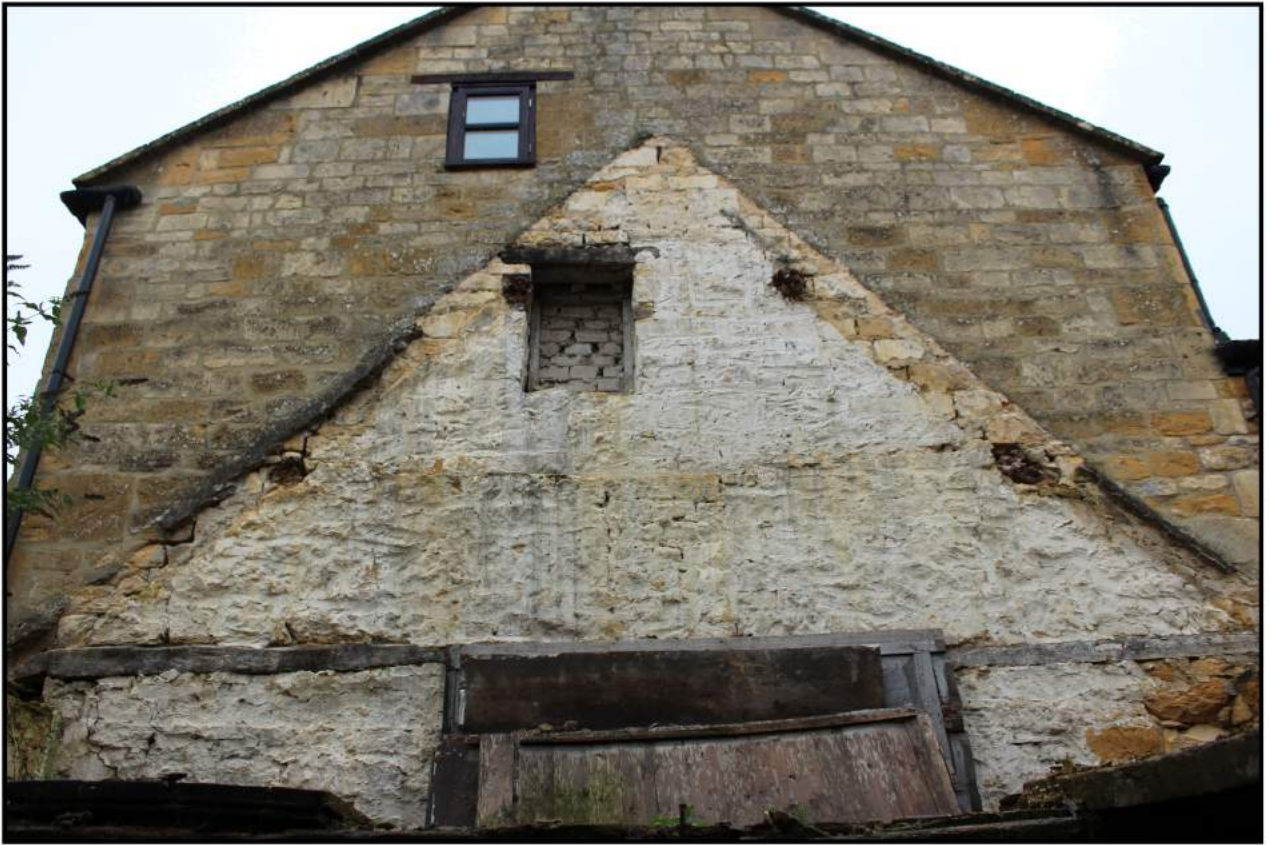
Fig 21: Scar on wall of building to south-west, showing blocked window and sockets for purlins
