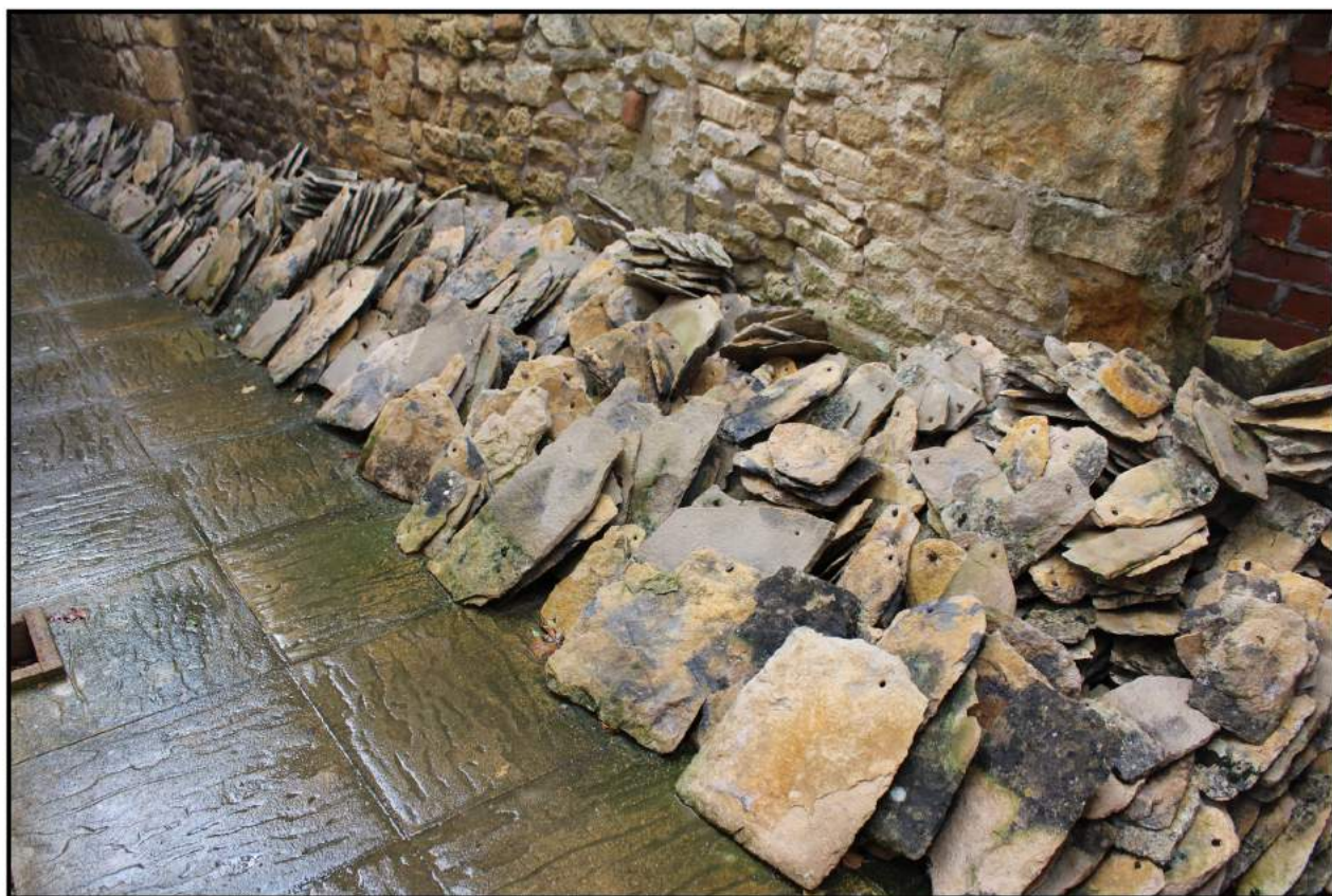
Fig 8: Stone tiles removed from collapsed roof
