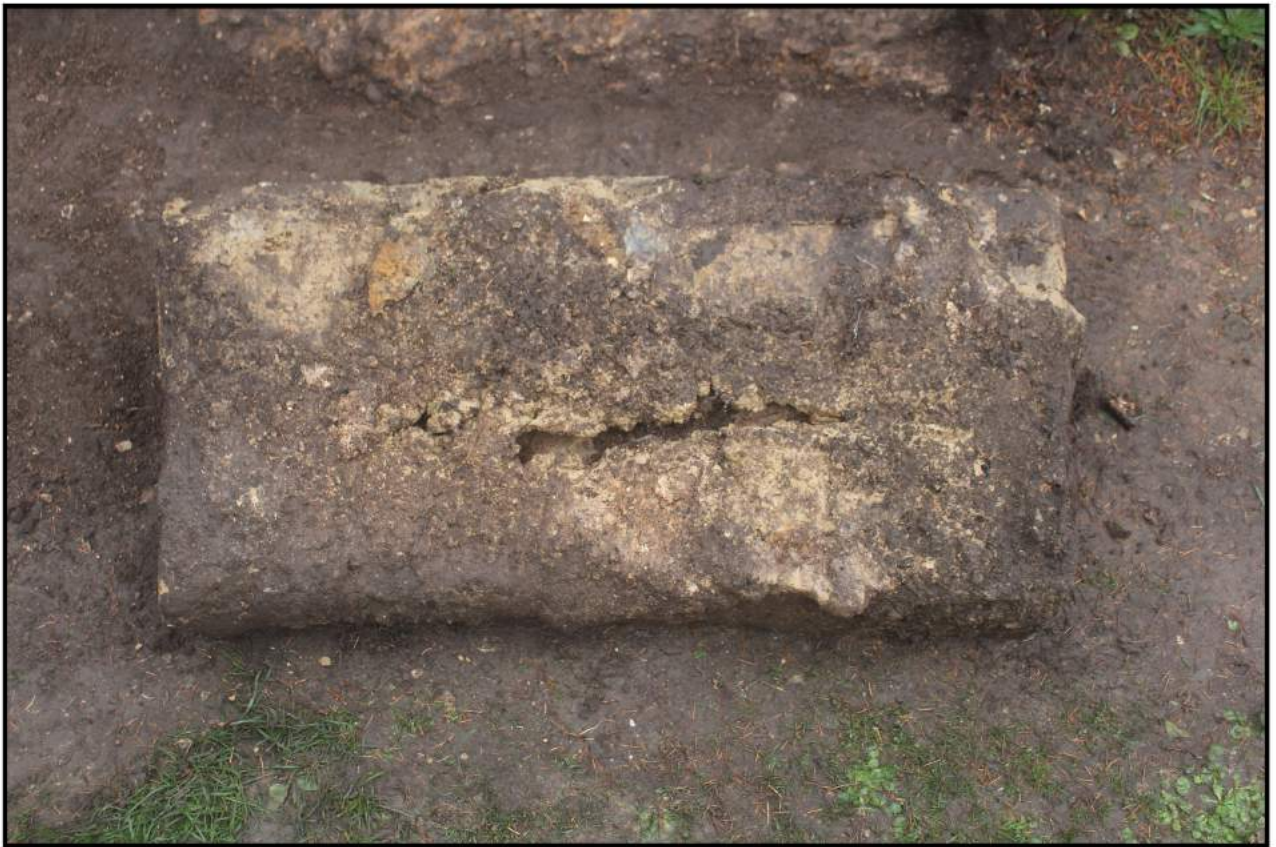
Fig 10: Underside of a step showing how mortar pushed underneath from the front and the back has left a gap near the middle
