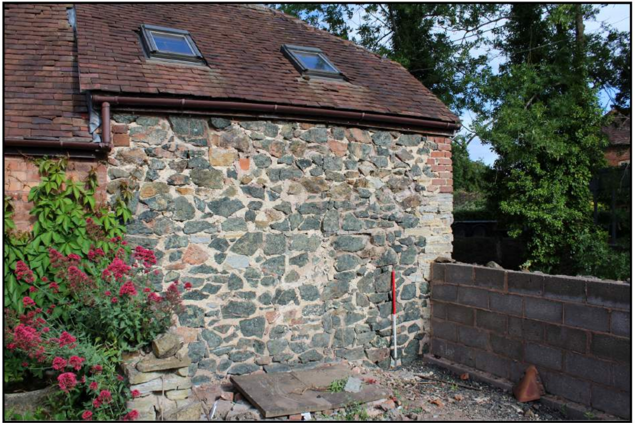
Fig 4: East wall of existing building showing part of south wall of sty and later block wall to north
