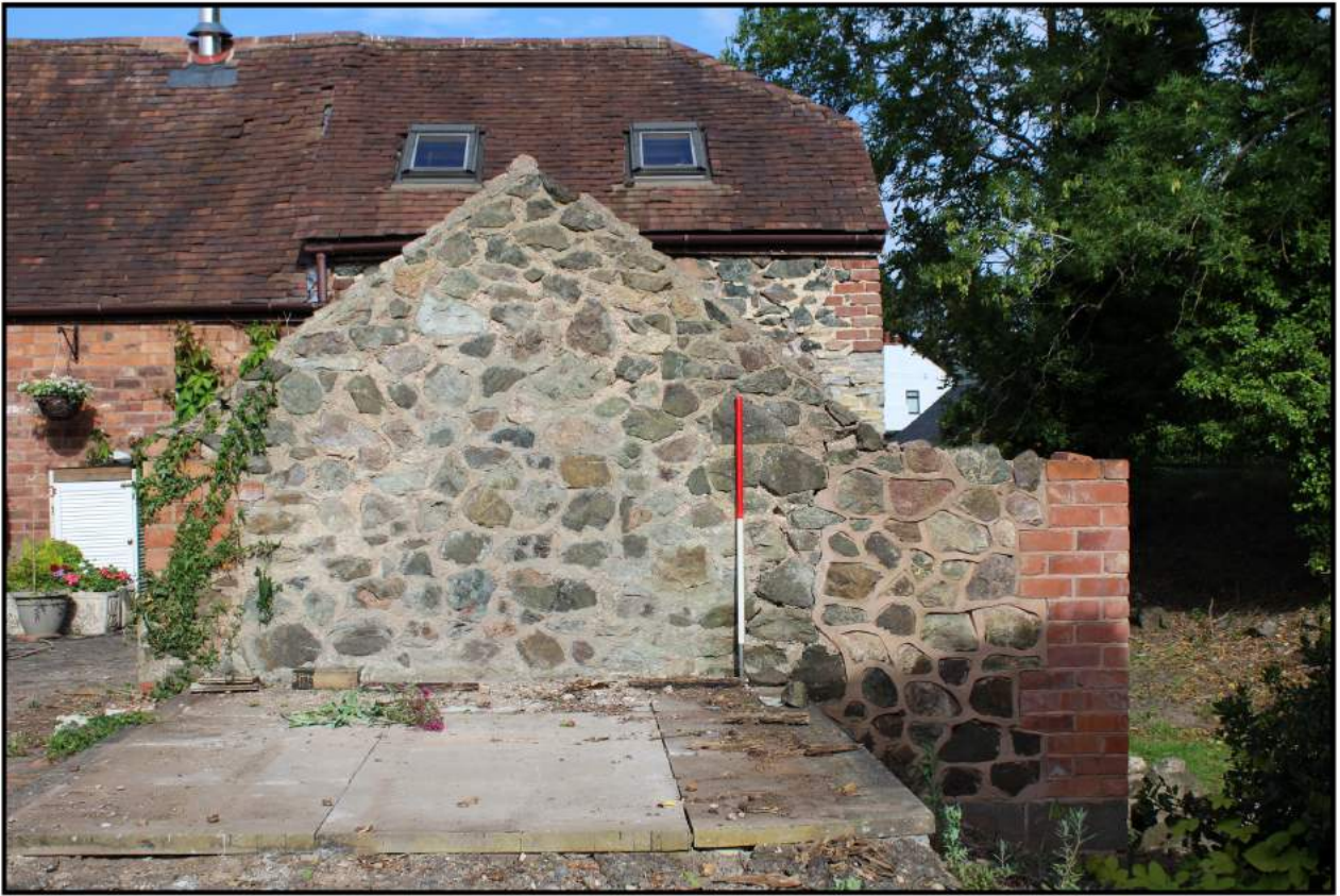
Fig 6: East wall of sty; east elevation showing later block wall faced with random stone
