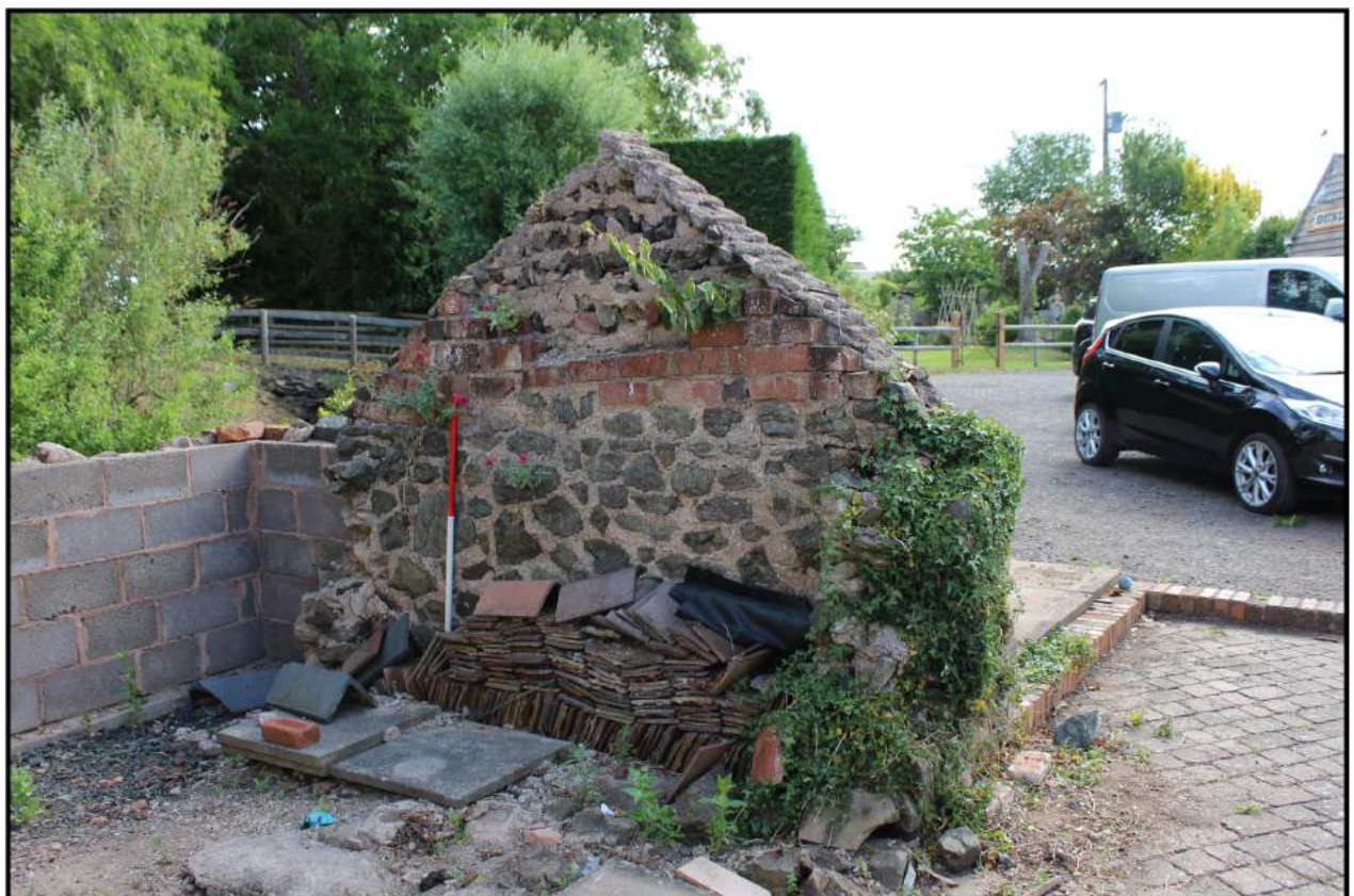
Fig 5: East wall of sty showing remains of original north and south walls and later block wall to north
