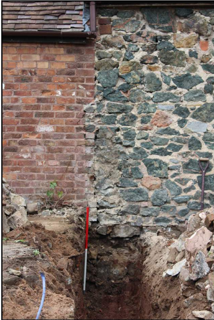
Fig 8: Southern footing trench and ghost of pig sty on wall of existing building
