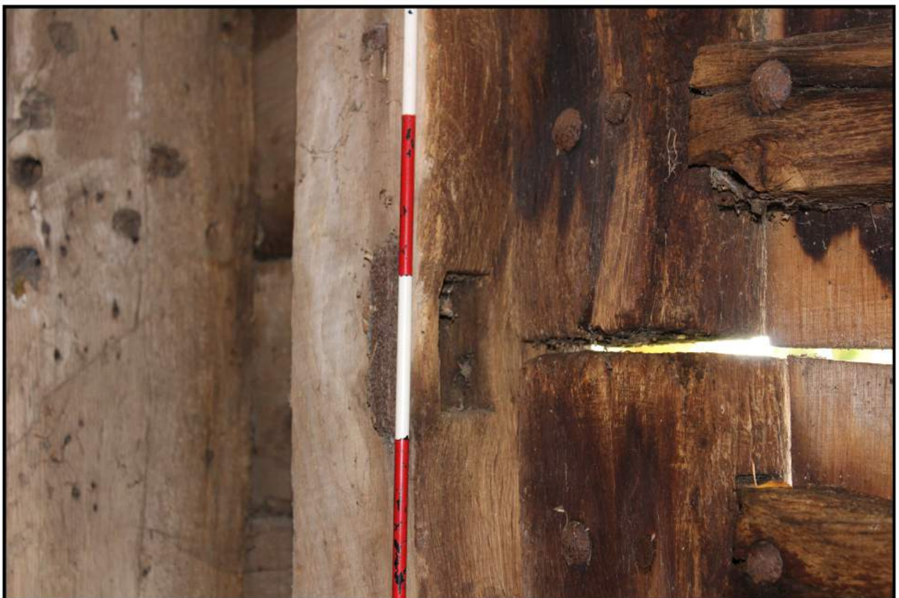
Fig 26: Barn interior; south-east elevation, adjacent to edge of threshing floor door, slot in post
