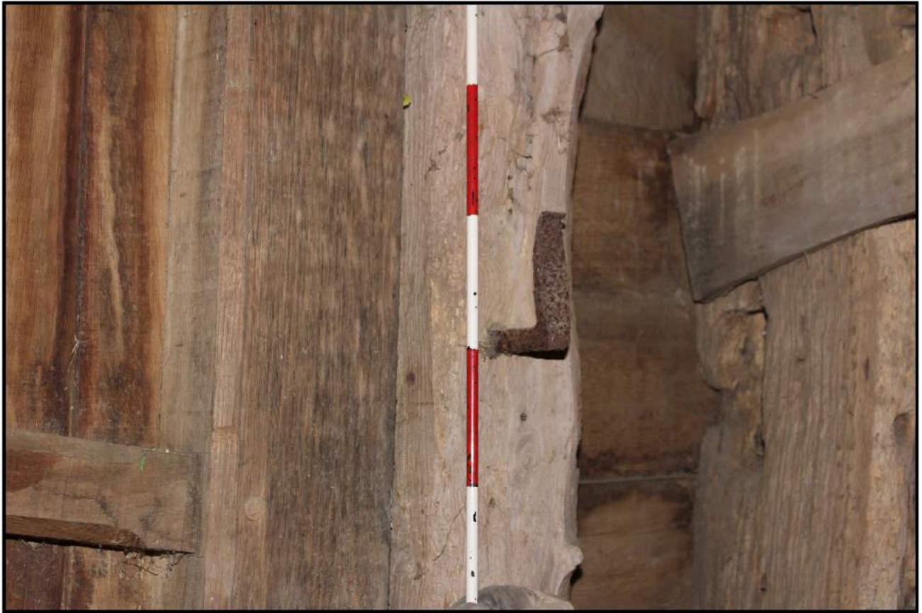
Fig 23: Barn interior; north-west elevation, adjacent to edge of threshing floor door, detail of metal fitting
