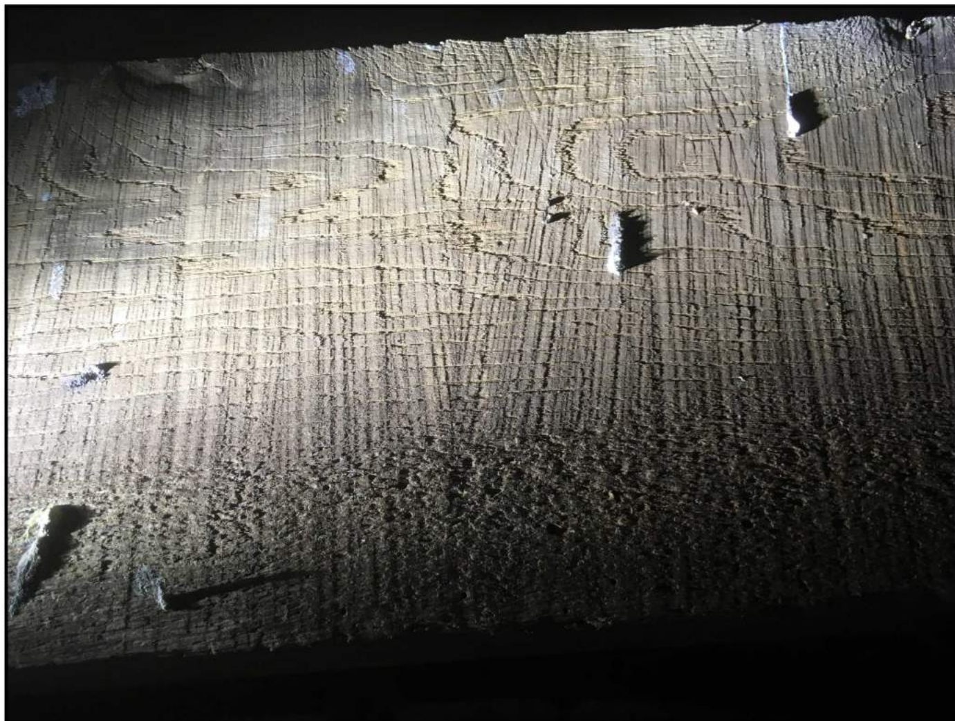
Fig 33: Straight saw marks on tie beam indicating that timber was 'pit sawn'
