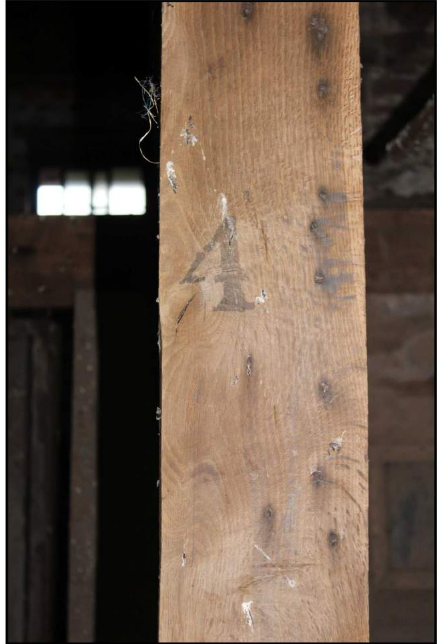
Fig 30: Stencilling on upper part of post
