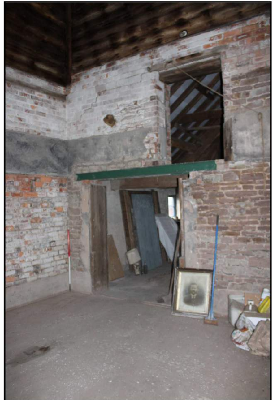
Fig 21: First floor, interior; showing sockets for floor joists and entrance to hop drying floor
