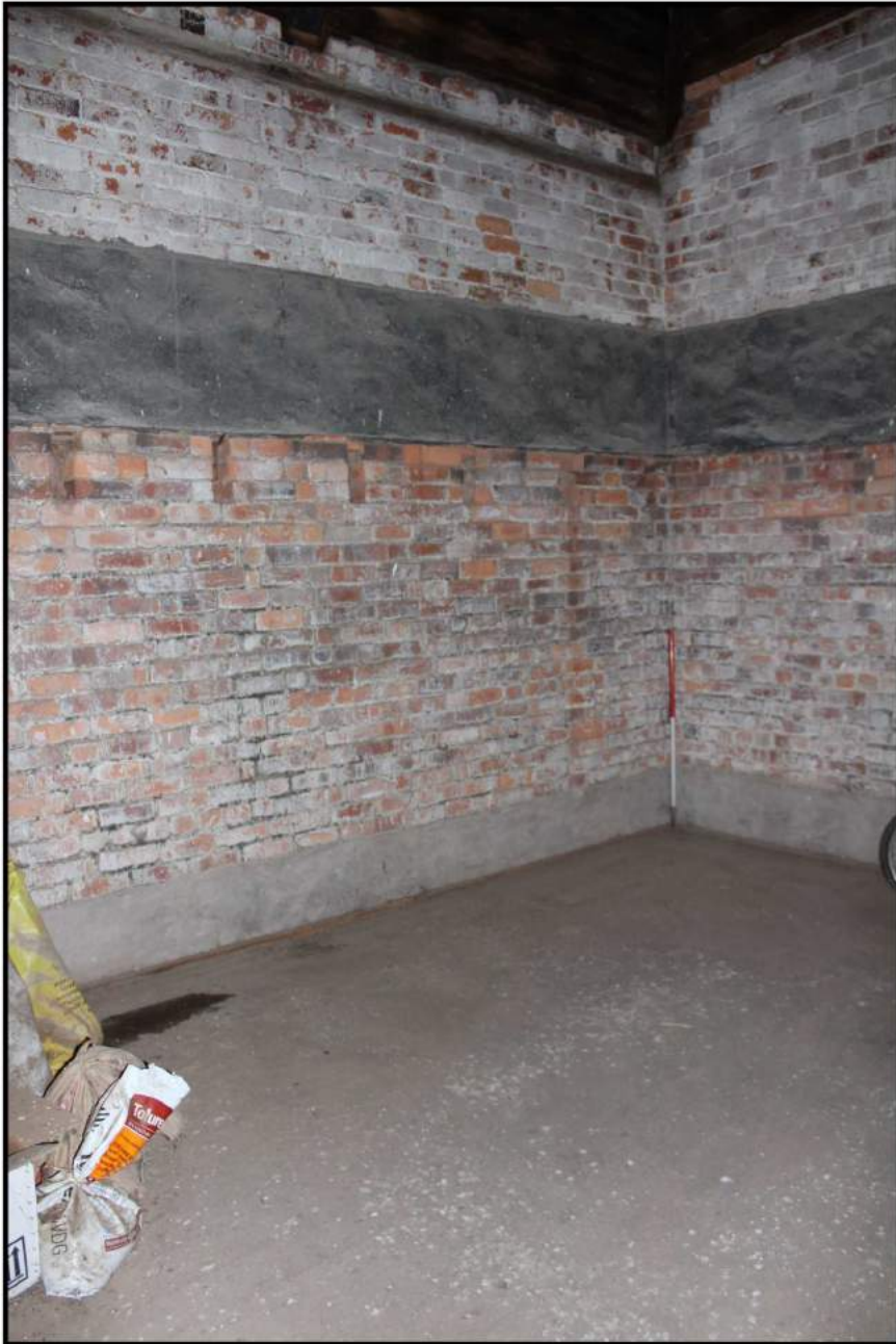
Fig 20: First floor, interior; showing sockets for floor joists that supported hop drying floor
