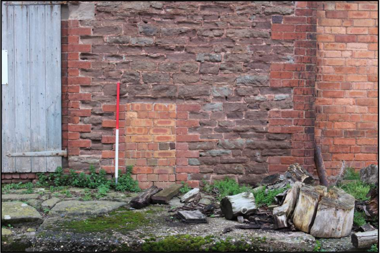
Fig 6: South-west elevation; detail of blocked opening
