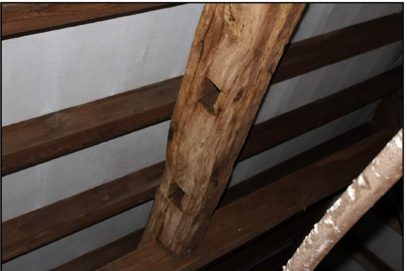
Fig 28: Detail of purlin; showing redundant mortices, indicative of former use as a floor beam
