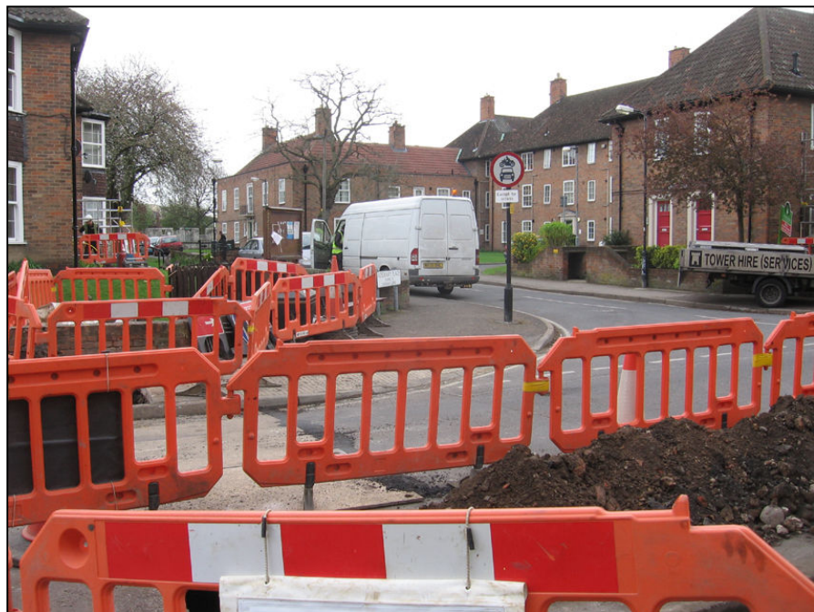
Plate 6 General view of works in progress at junction of Navigation Road And Rosemary Place, looking east
