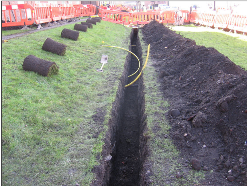
Plate 1 General view of main trench in lawn at northern end Of Navigation Road, looking south-west
