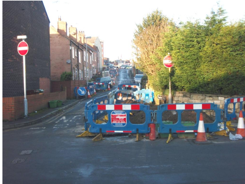
Plate 1 View of the works along Thackray Lane from the bottom of the lane, looking north-west
