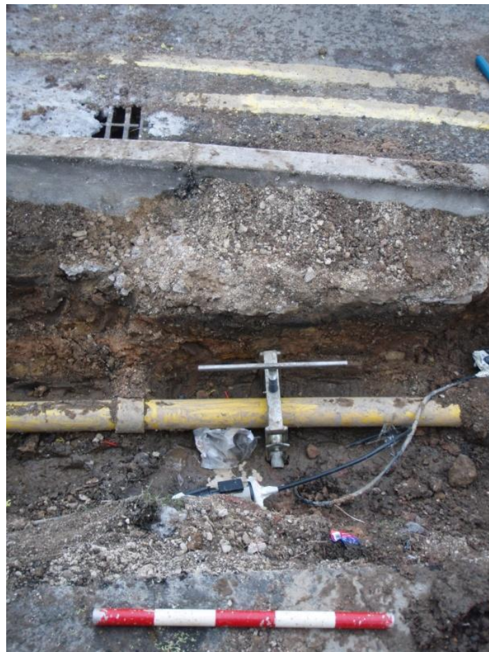
Plate 36 The central portion of the east facing section of Trench 29 facing west, showing the sandstone visible at the base of the section, scale unit 0.1m.
