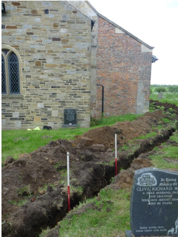
Plate 10 Looking west along line of wall 1005, showing northern wall-line of former chancel
