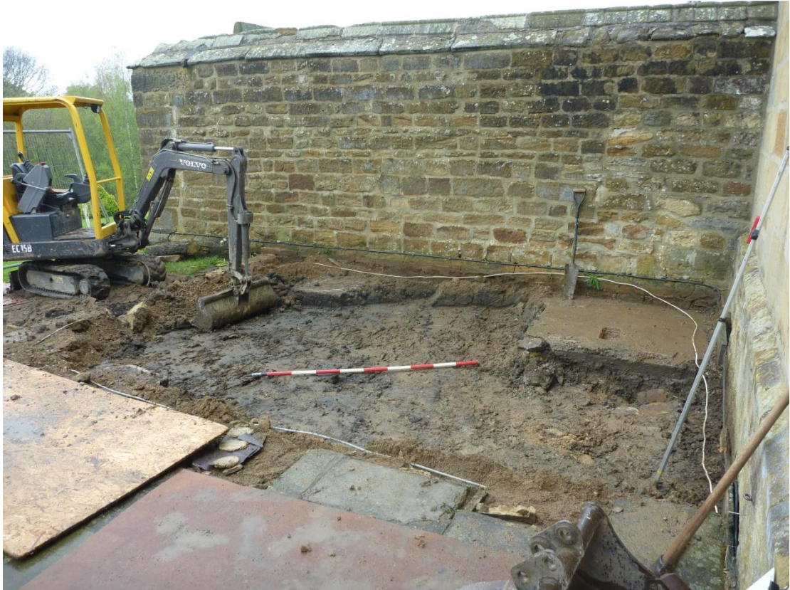
Plate 2 View of works for library extension. Note concrete setting to NW corner and two concrete settings for posts (on line with mini-digger bucket). Looking SW.
