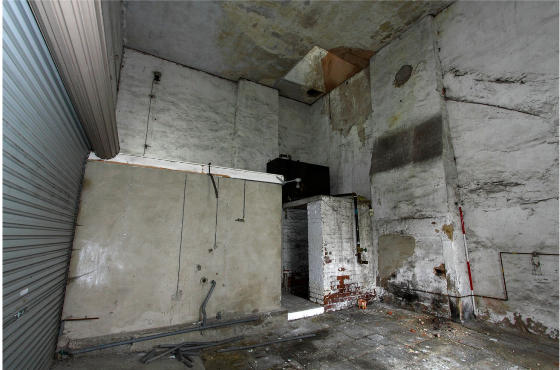
Plate 25 W and S walls of Brewhouse interior, looking SW. Note inserted garage door and bathroom to left. Square section wooden pipe with fitting below in upper left.
