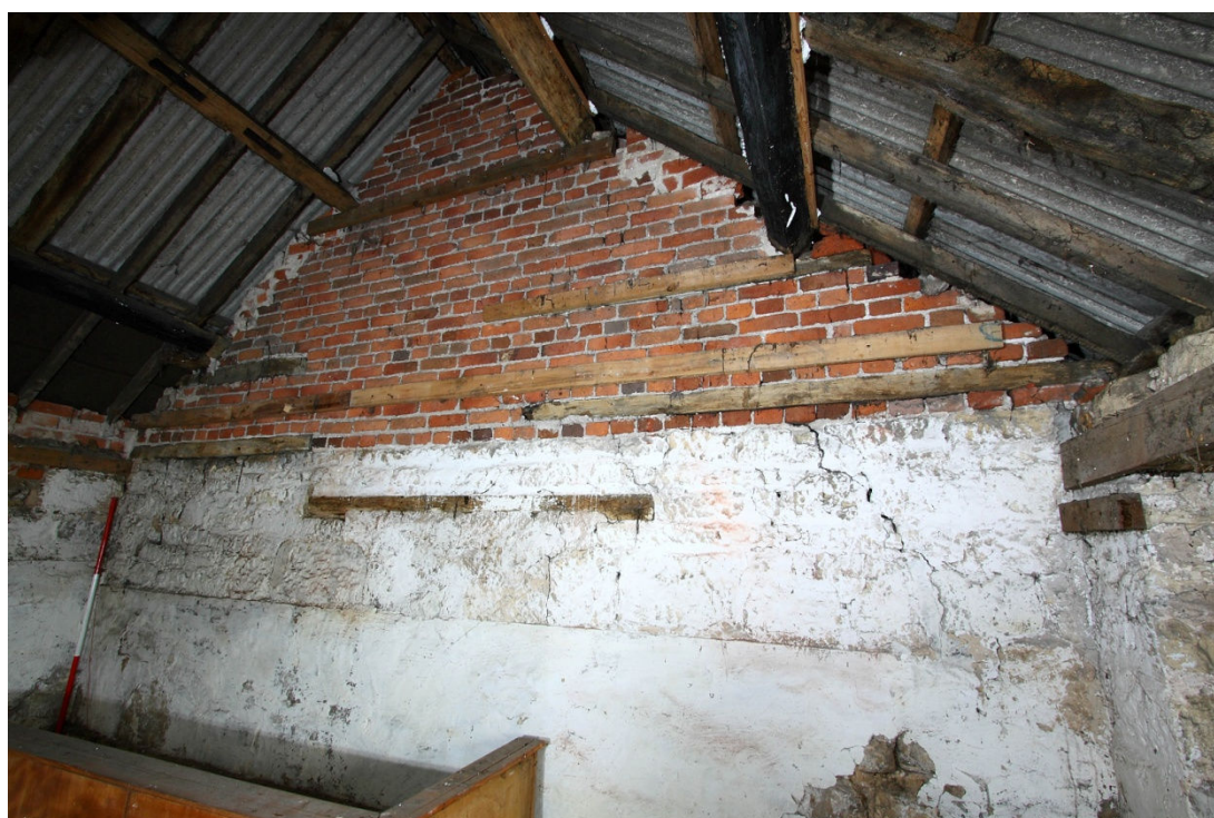
Plate 10 Later brickwork of gable end (formerly hipped) of W end of original building of south range, looking W (note timber lintel of blocked early first floor doorway)
