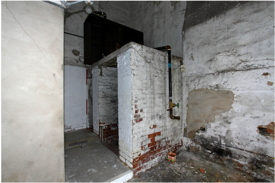
Plate 27 Fuel-store within Brewhouse interior, looking SW. Tank above is for storage of oil for Aga.
