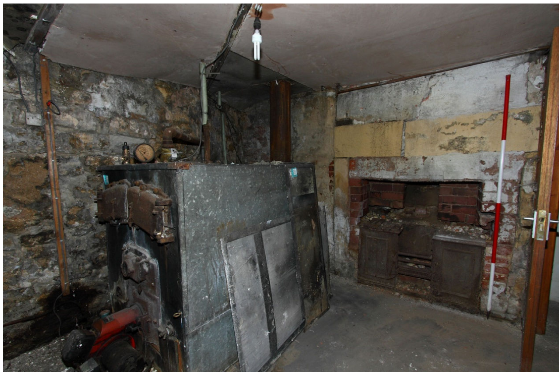
Plate 8 Boiler room of early building of south range, note succession of fireplaces, looking E
