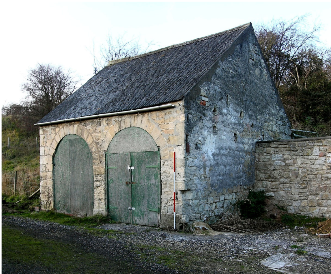
Plate 14 Cart shed with dovecote over, looking NW. (Note roofline of former structures in gable end to right)
