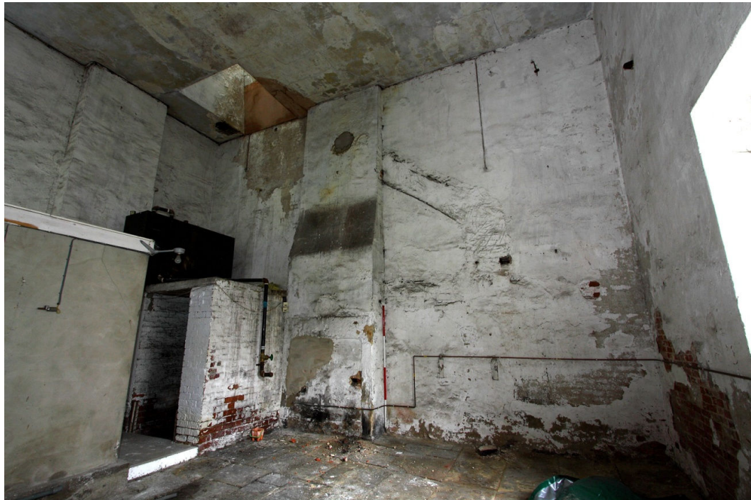
Plate 24 W wall of Brewhouse interior, looking W. Note tapering hood to upper left, blocked up fireplace and scar of old flue to right of extant flue. Small pulley wheel is present to upper walling to right and to left of this a high level iron fitting.
