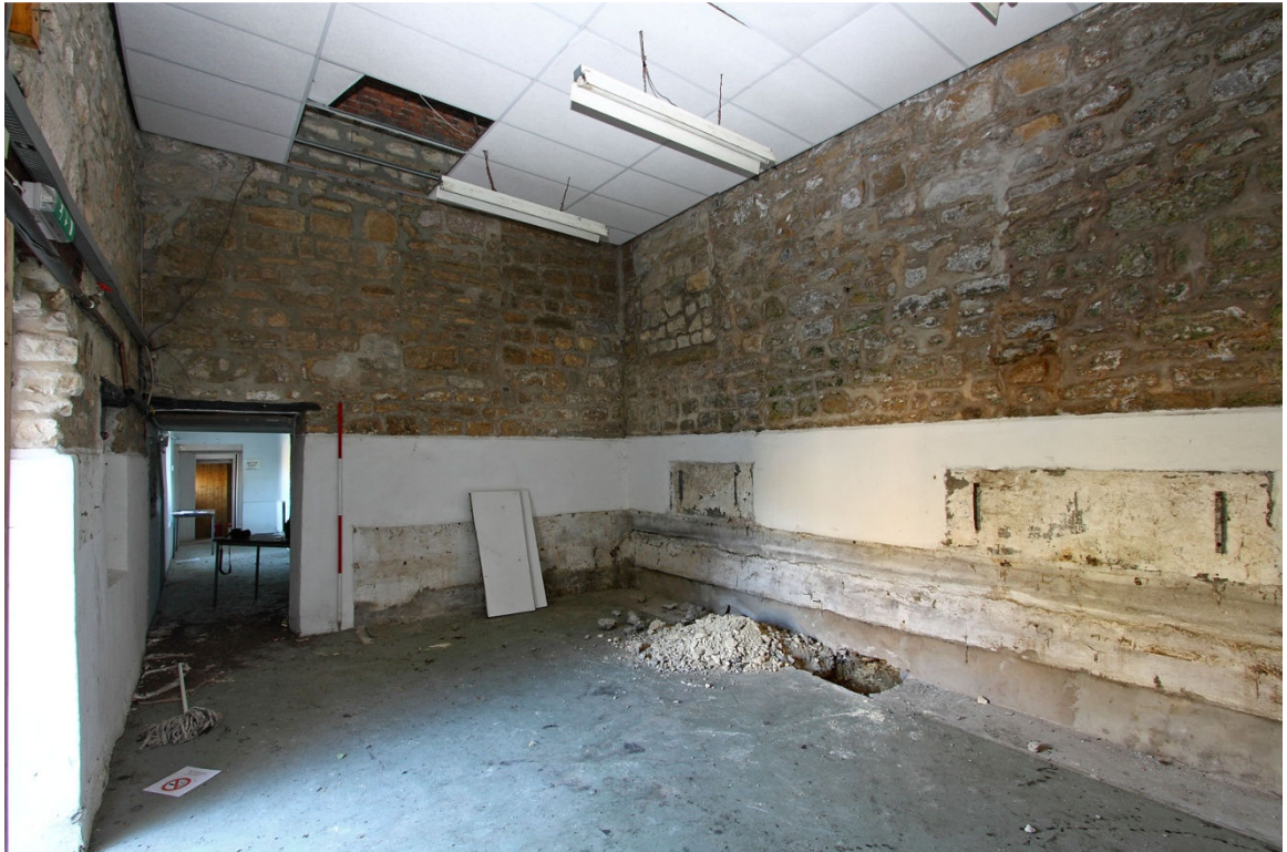
Plate 13 Infill building of south range, looking E. (Note blocked openings to right)
