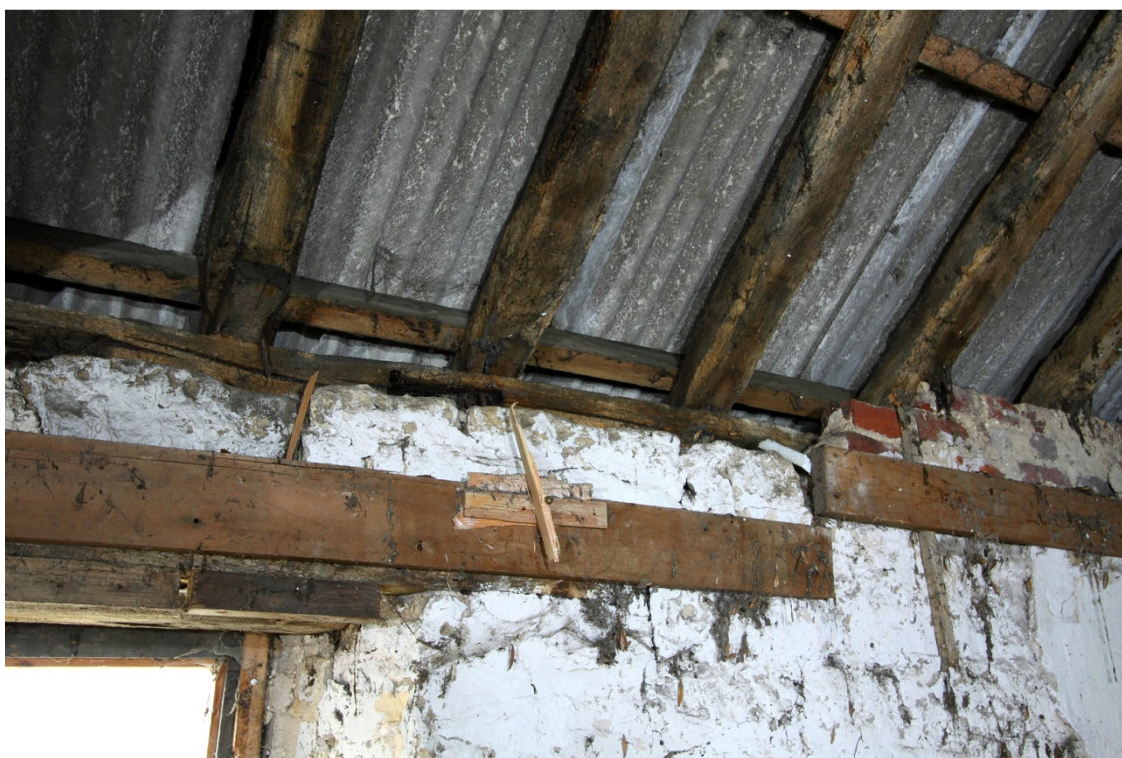
Plate 12 Rafters of original building of south range resting on wall plate, looking N
