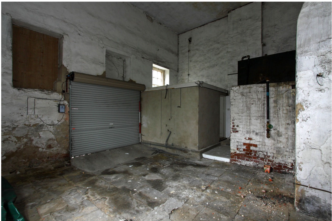
Plate 26 S and E walls of Brewhouse interior, looking SE. Note modern inserted garage door and bathroom.
