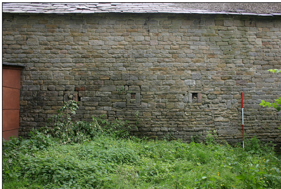
Plate 14 Building A2, north elevation showing different build on upper and lower sections of wall
