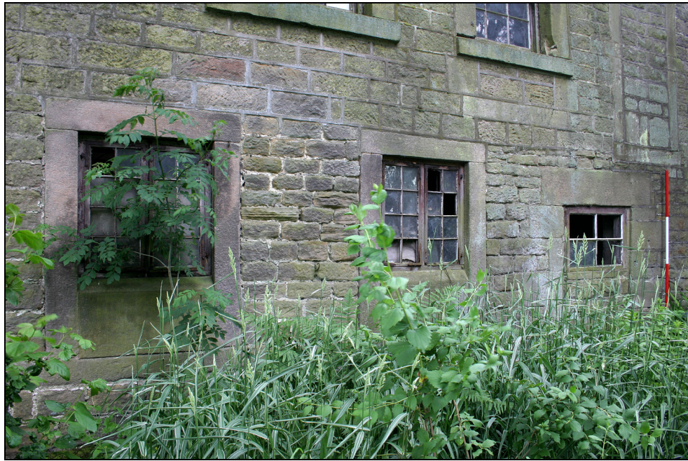
Plate 16 Building A3, north elevation, showing differential build between upper and lower sections
