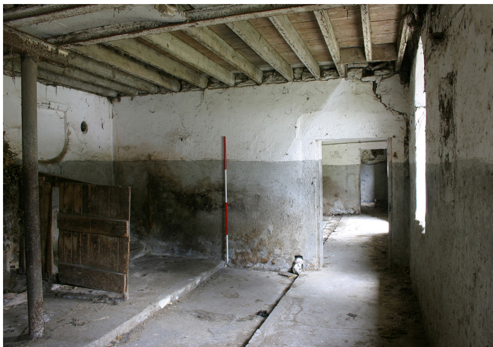
Plate 12 Building A2, wooden shippon and recessed feeding niches in rear wall, facing east
