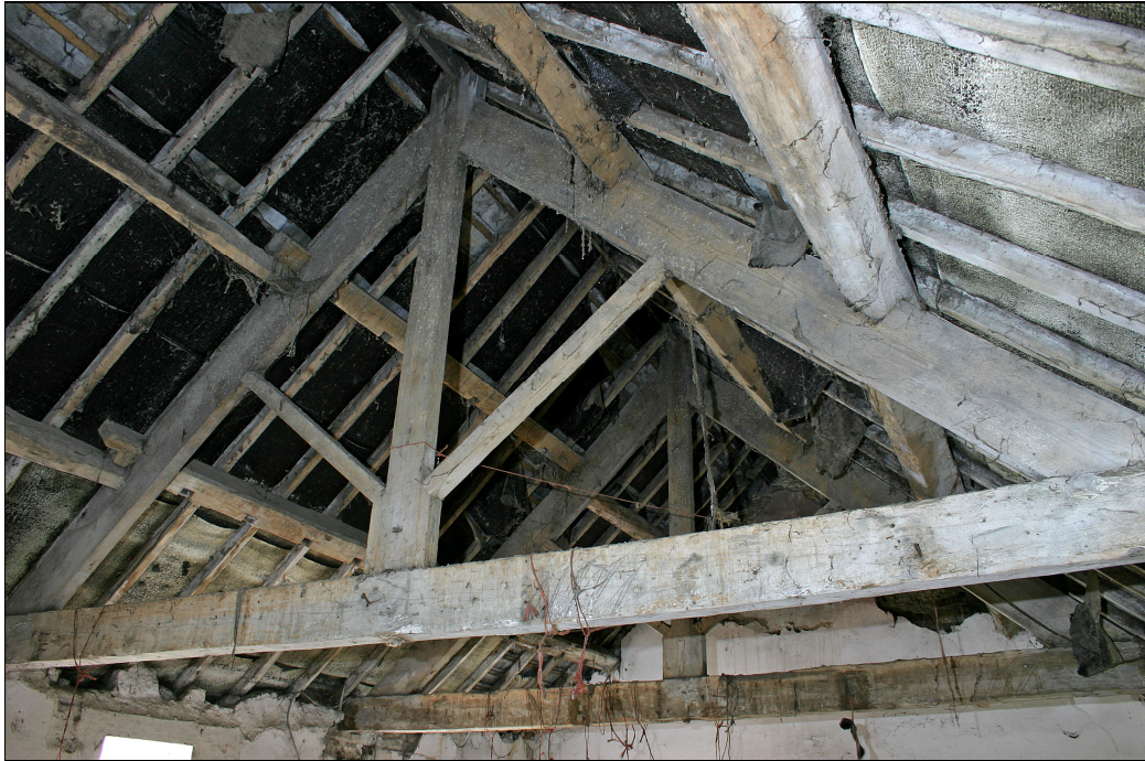
Plate 20 Building B, first floor interior, detail of roof (Note re-used purlins on far side)
