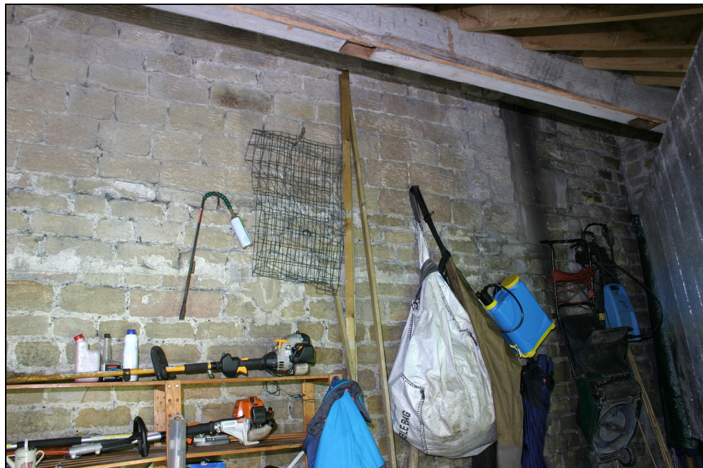
Plate 17 Building A4, north elevation, first floor quoining for A2 visible at the dark patch to right and different build between upper and lower parts of wall identifiable
