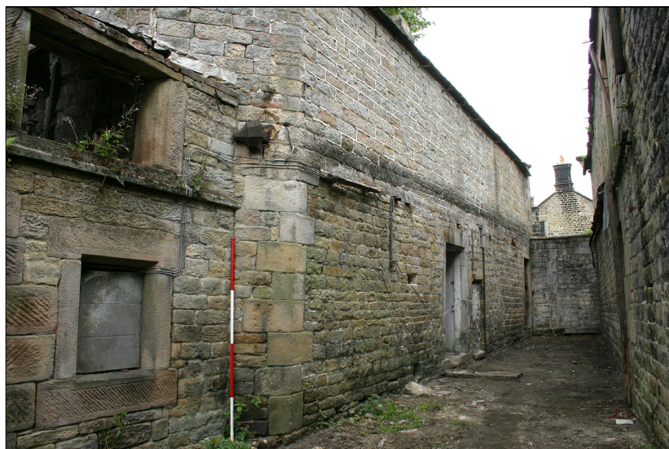
Plate 15 Building A3, south elevation, showing single storey coining and differential build between upper and lower sections of wall
