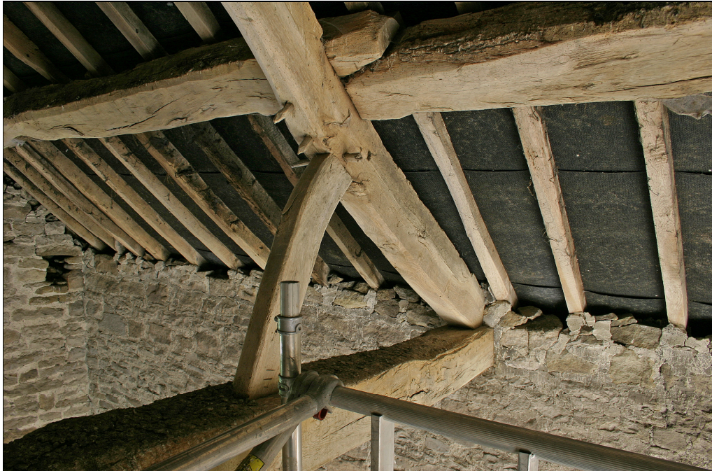
Plate 25 Building C, detail of roof truss (Assembly marks visible to left of scaffold where the queen strut meets the tie beam)
