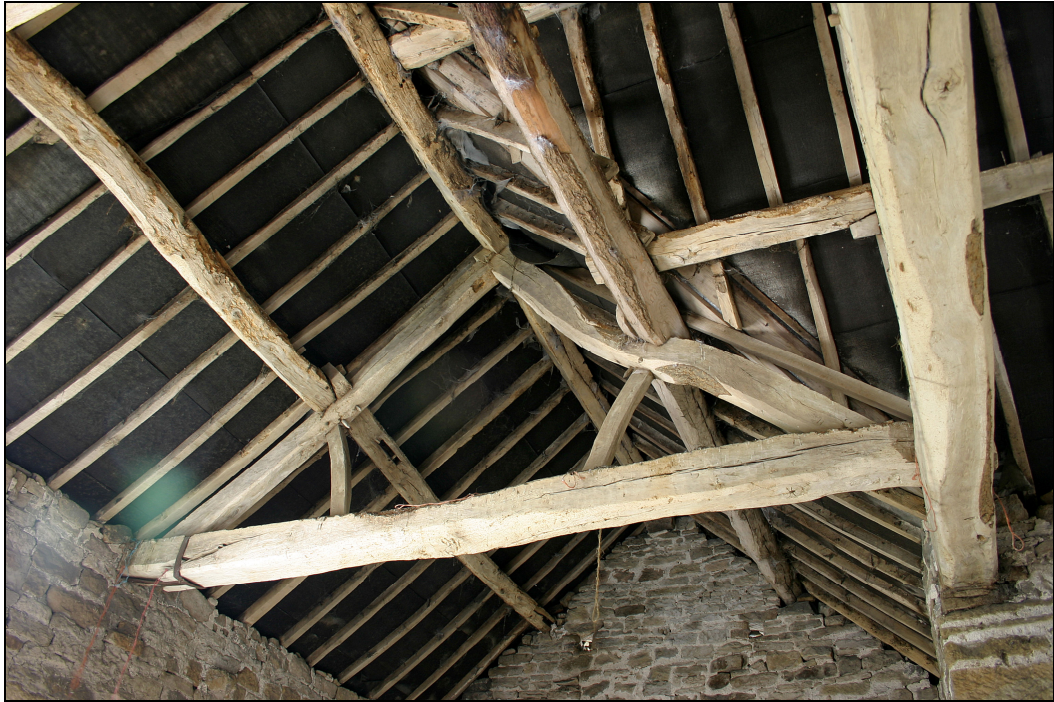
Plate 26 Building C, arrangement of trusses where the cross wing meets the main axis, facing north
