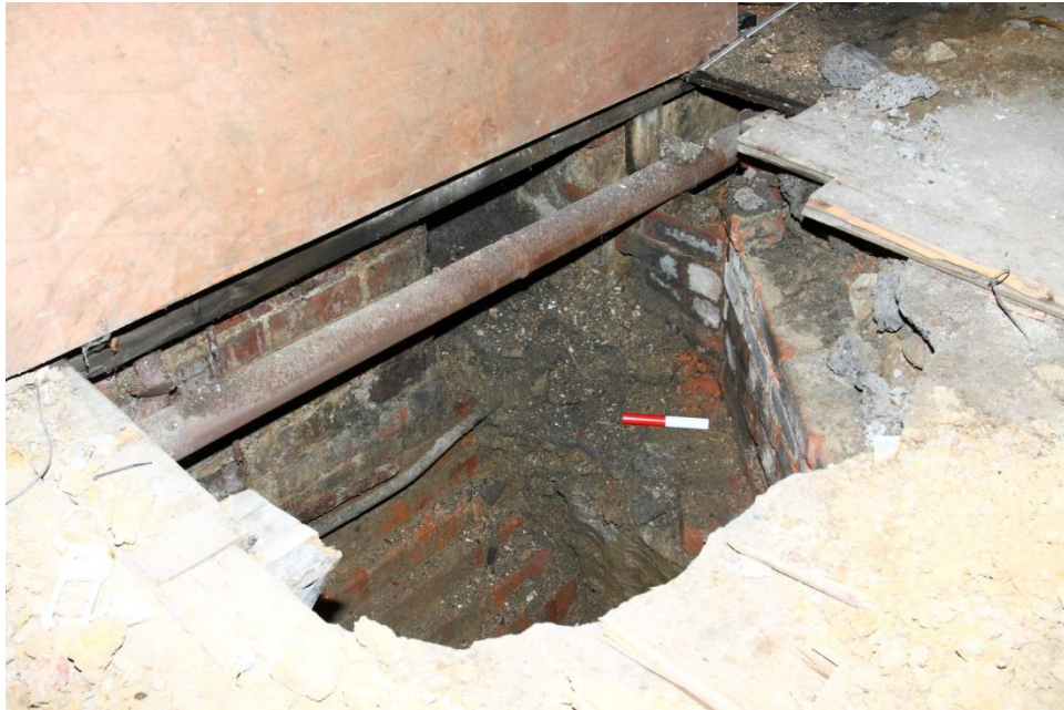
Plate 7 Test-pit to S. internal corner area of the cinema, looking S. Note the pipe duct, offset footings, basal part of wall vent and brick lined end of 'sub-floor duct' (78jpg)
