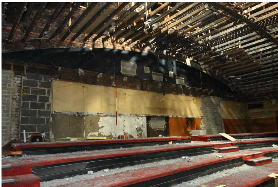
Plate 11 Rear wall of the circle showing blocked up openings, looking E. (42jpg)
