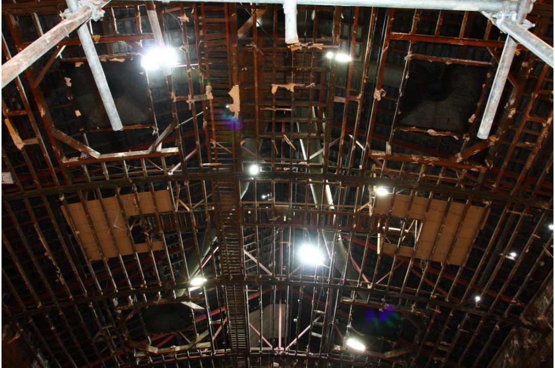
Plate 16 General shot of the ceiling and roofing arrangements above the auditorium, looking S.W. (30jpg)
