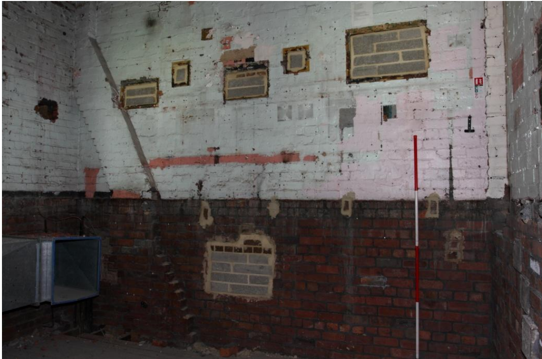
Plate 23 The S.W. wall of the projection room, looking S. Note the chimney flue and blocked apertures.(the lower blocking is not understood, there is no corresponding scar within the circle and it does not appear on any plans) (70jpg)
