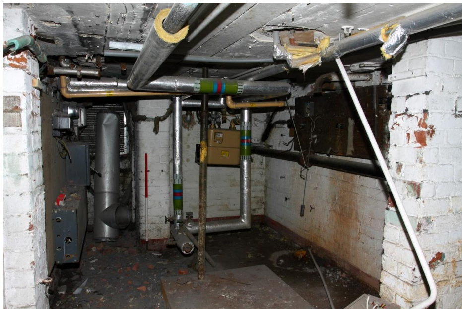
Plate 18 The S.E. chamber of the basement, looking S.E. Note switchgear, note water pipes, gas meter and mounting block. (60jpg)
