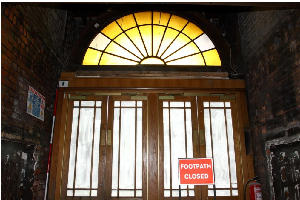
Plate 20 Entranceway to the foyer, looking S.E. Radiator recesses can be seen to either side. (55jpg)
