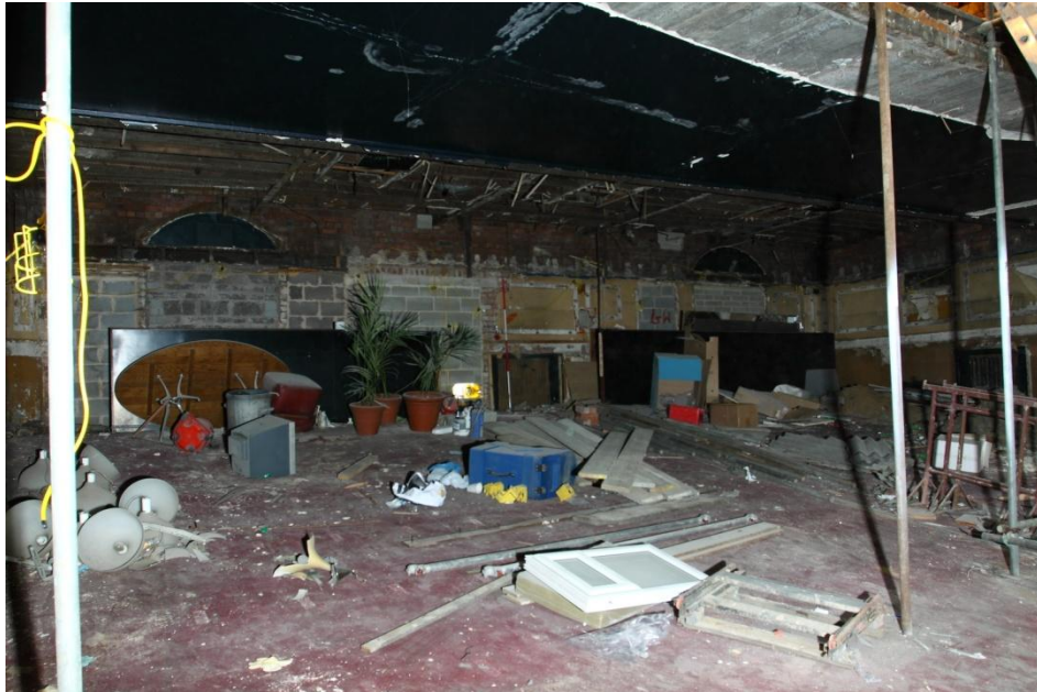
Plate 10 N.E. 'back' wall of the auditorium, looking E.N.E. The blocked up doorway to the foyer not shown on any plans lies immediately left of the ranging rod. (29jpg)
