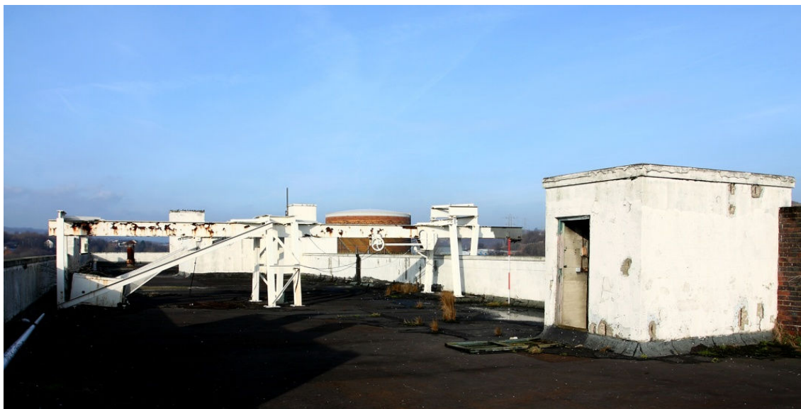
Plate 20 Beam crane on roof, looking NW
