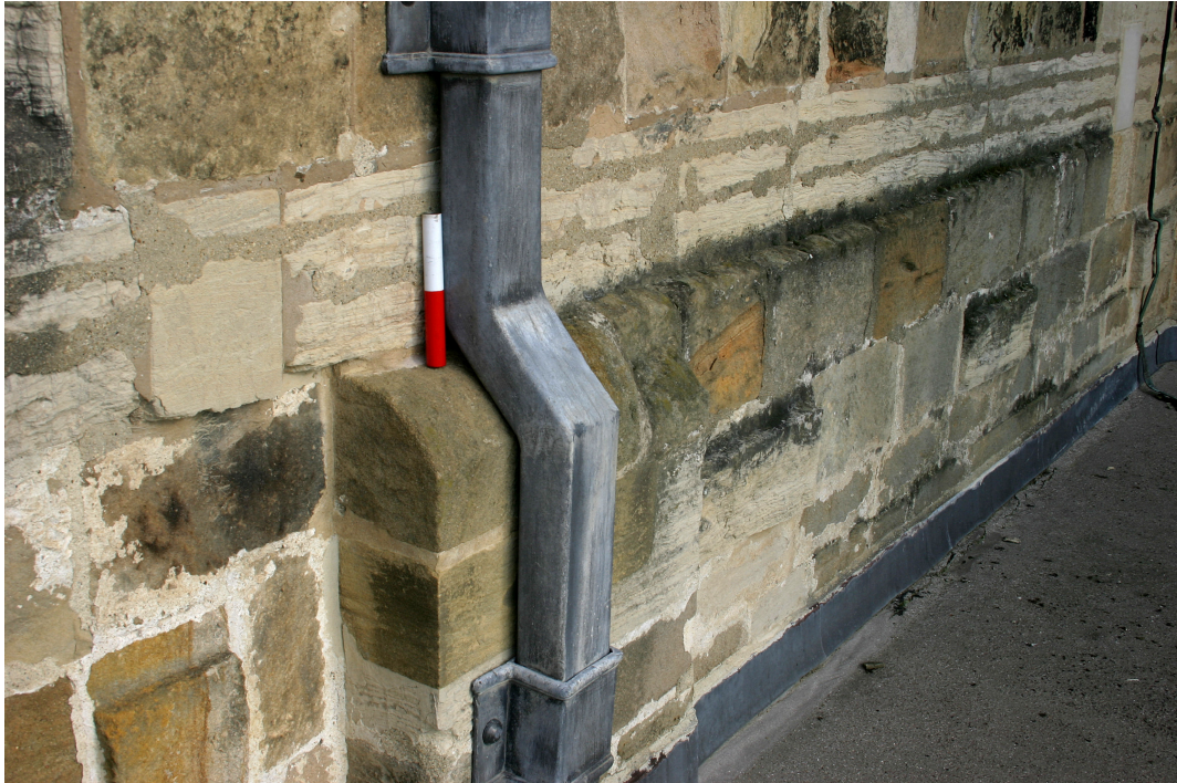
Plate 1 Scars of the original roof-line on the south face of the nave walling, behind the scale. Scale in 0.10m units
