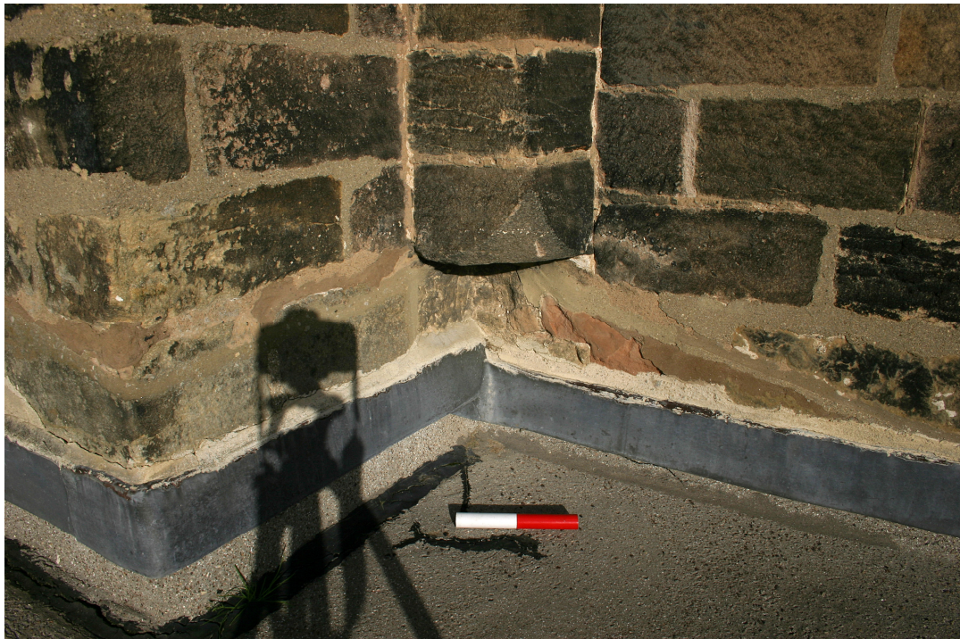
Plate 3 Cushion moulding to base of vertical order. This order appears to have been truncated in order to ease fitting of the roof to the south aisle at the time of its construction.
