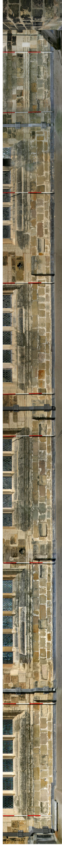
View of entirety of nave walling at level of south aisle roof, compiled from a composite of digitally rectified photographs. Scale in 0.5m units
