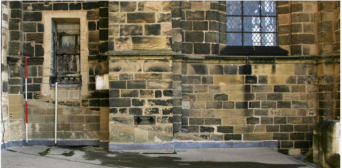
Plate 4 View of the W side of the south transept showing roof scar of original south aisle roof, the contemporary inserted doorway and cushion moulding to vertical order – immediately to right of buttress. Scale in 0.5m units
