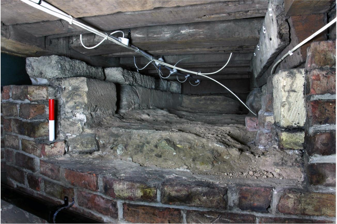
Plate 7 East side of N. line of early walling, looking ENE. Note the mortar surface in front of walling. Stonework above the walling forms propping for beam of choir stalls
