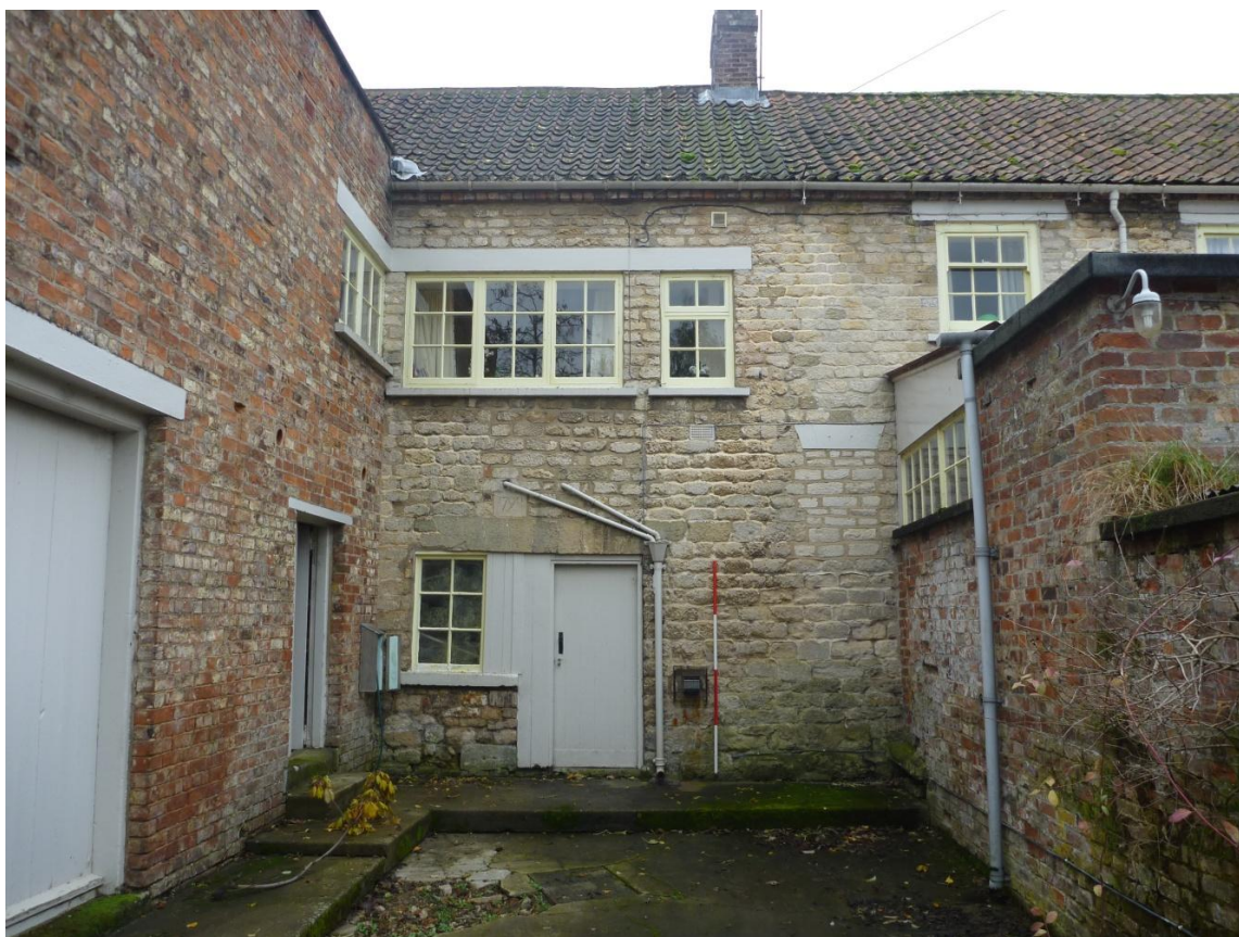
Plate 9 View of the rear of mill showing the narrowed original entrance with date-stone above and brick extension to left. Parts of the brick wall to the right once formed part of an extension also. Note the blocked-up window to the mill house and later windows at first floor level within the mill.
