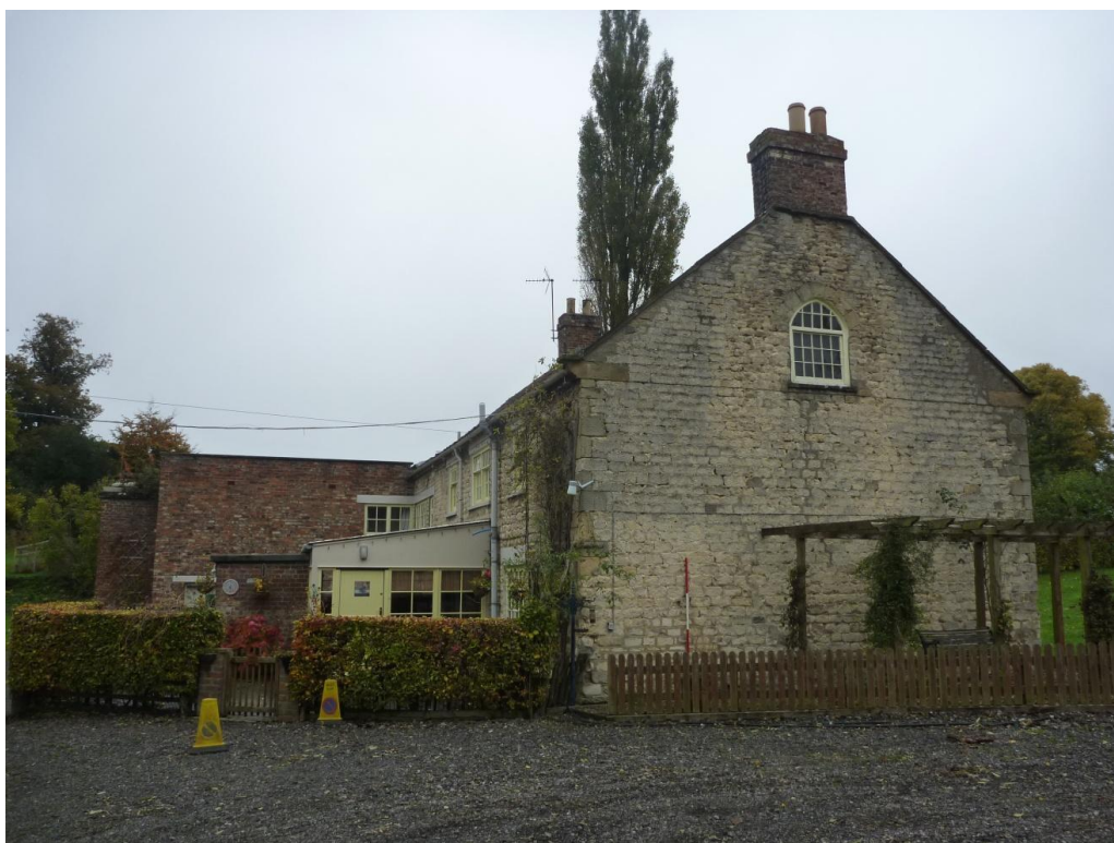
Plate 7 End (SW) elevation of Mill House. Note the truncated remains of the brick extensions including chimney.
