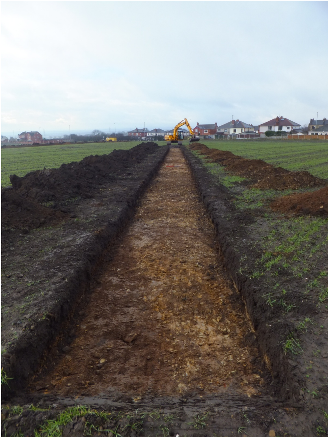
Plate 15: Example of bedrock natural exposed in the base of trench 29 (south facing).
