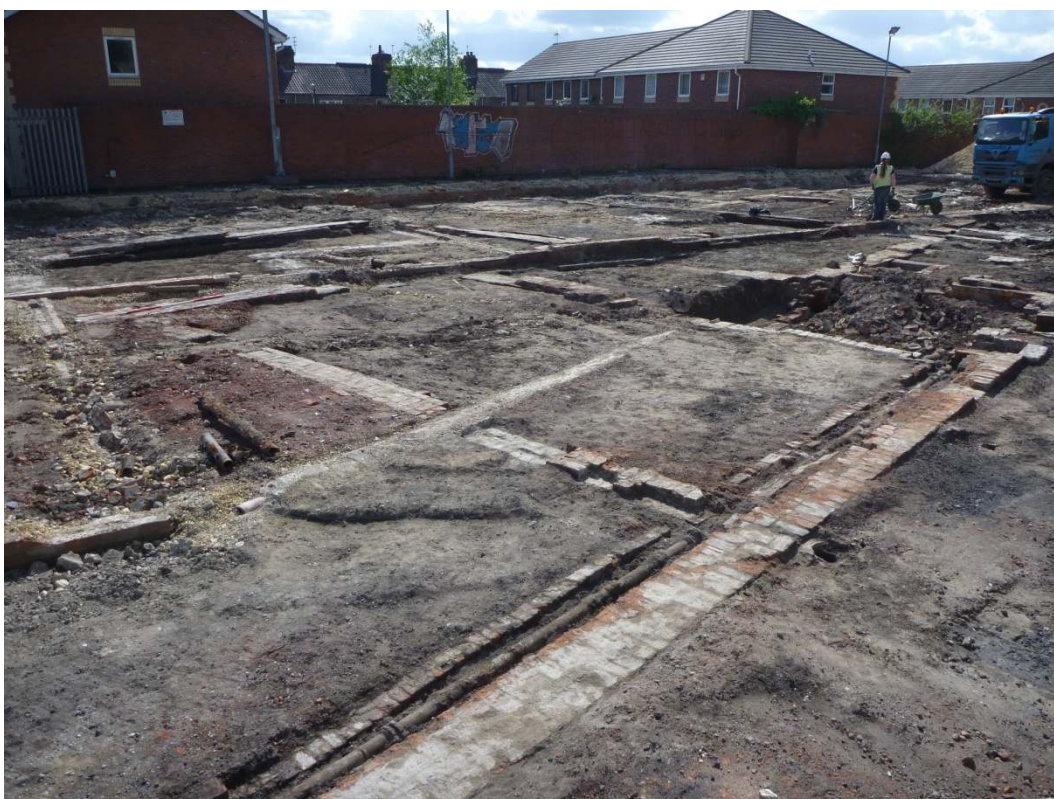
Plate 2: Working shot of St. Lawrence School and Bootham works viewed from the north.
