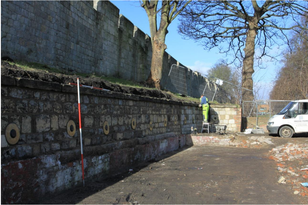
39. West facing view of the retaining wall during restoration. Scale units 0.5m
