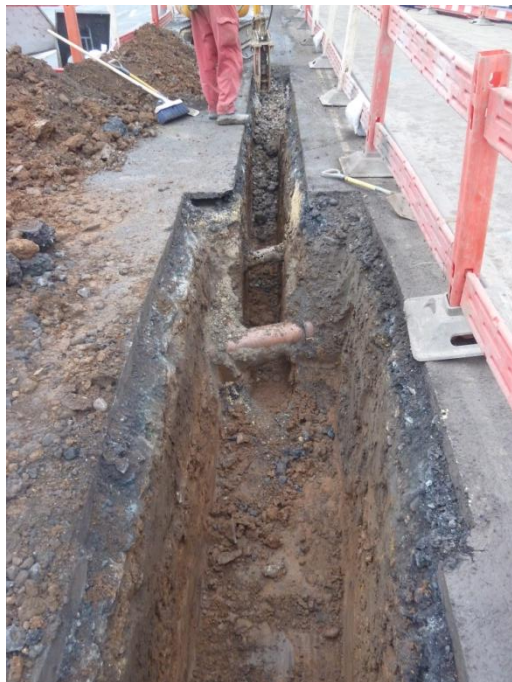
Plate 2. West end of Hydrant pit and start of utility trench looking W
