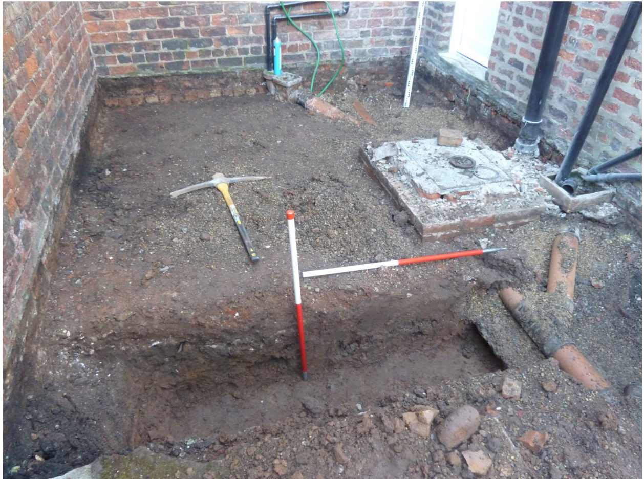
Plate 2. Trench looking ESE showing modern services and excavated foundation trench for conservatory wall. Scales- 1m in 0.5m divisions
