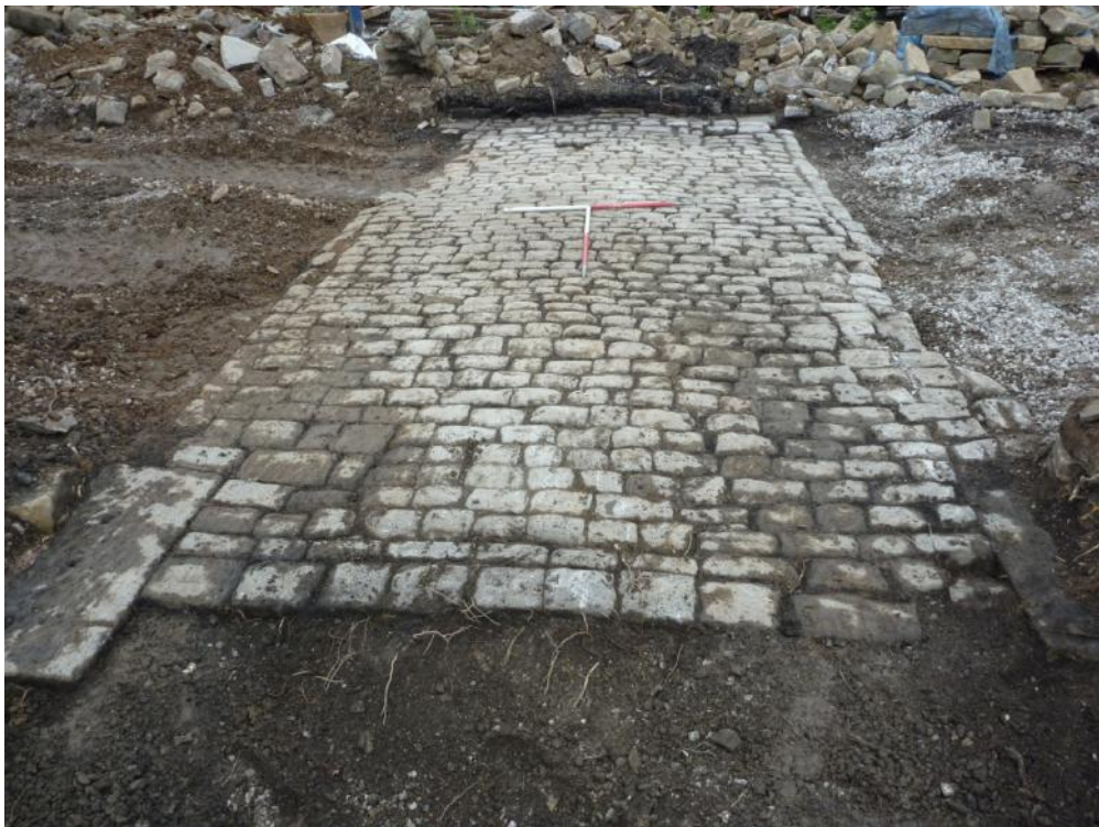
Plate 9 Track way, Building 6 before new foundations cut. Western entrance In foreground. 0.50m scale divisions.
