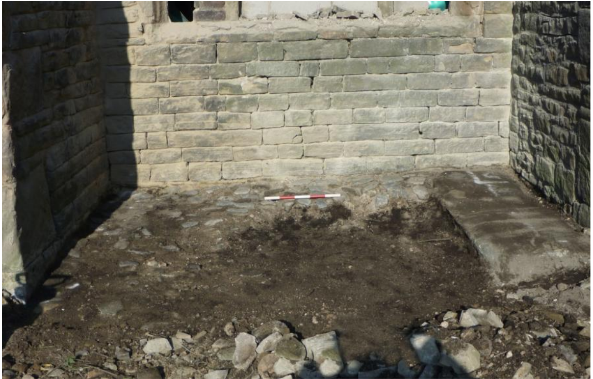
Plate 20 Trench 30 showing extent of damage suffered between 2003 and 2012. Looks north-west. 0.10m scale divisions.
