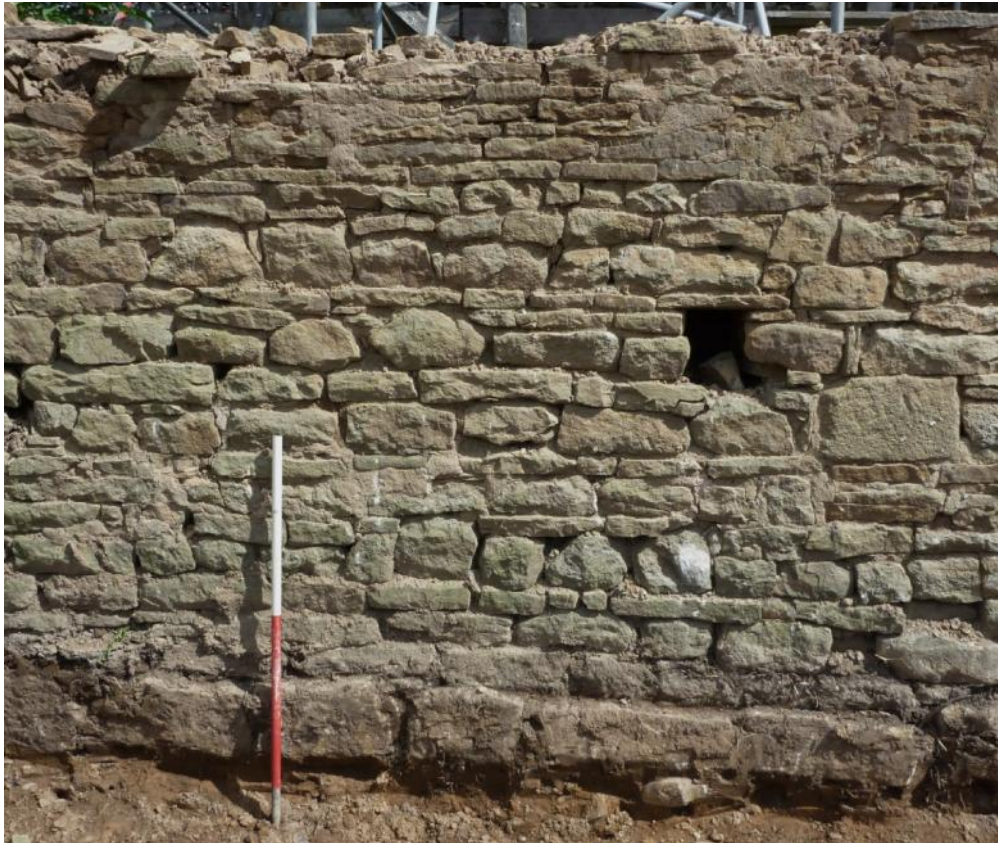
Plate 25 Part demolished northern wall of Building 6 showing elevated single course foundation above depth of internal floor reductions. 0.50m scale divisions
