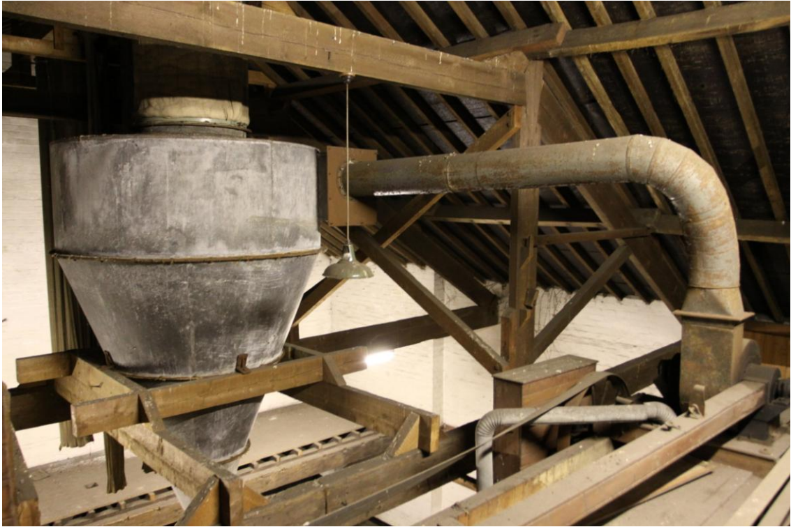
Plate 39: Pipe attachment from Dressing Machine to Hopper, 3 rd Floor Level (Photograph 202).
