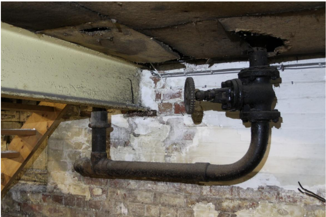
Plate 30: Outlet Pipe and Stopcock for Steeping Cistern Ground Floor Level (Photograph 53).
