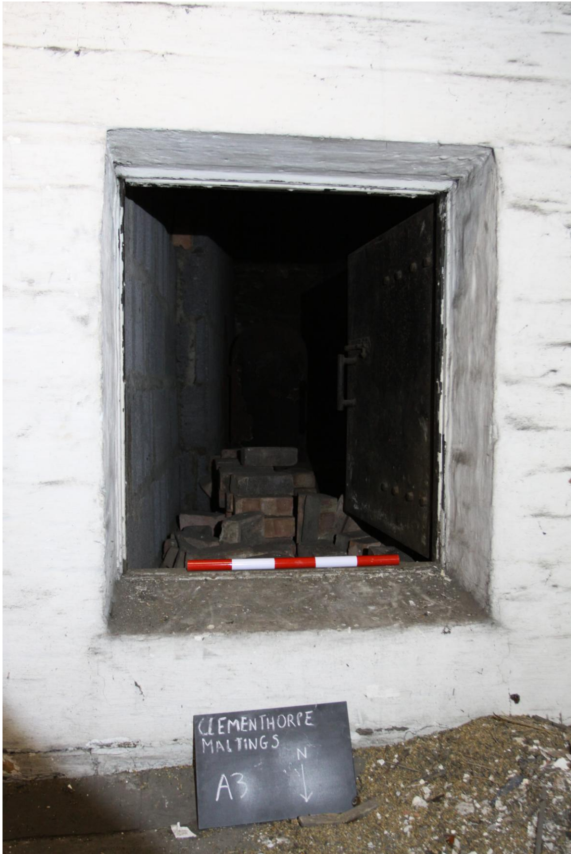
Plate 8: 2 nd Floor Level Doorway into the underside of the kiln drying floor (Photograph 195).
