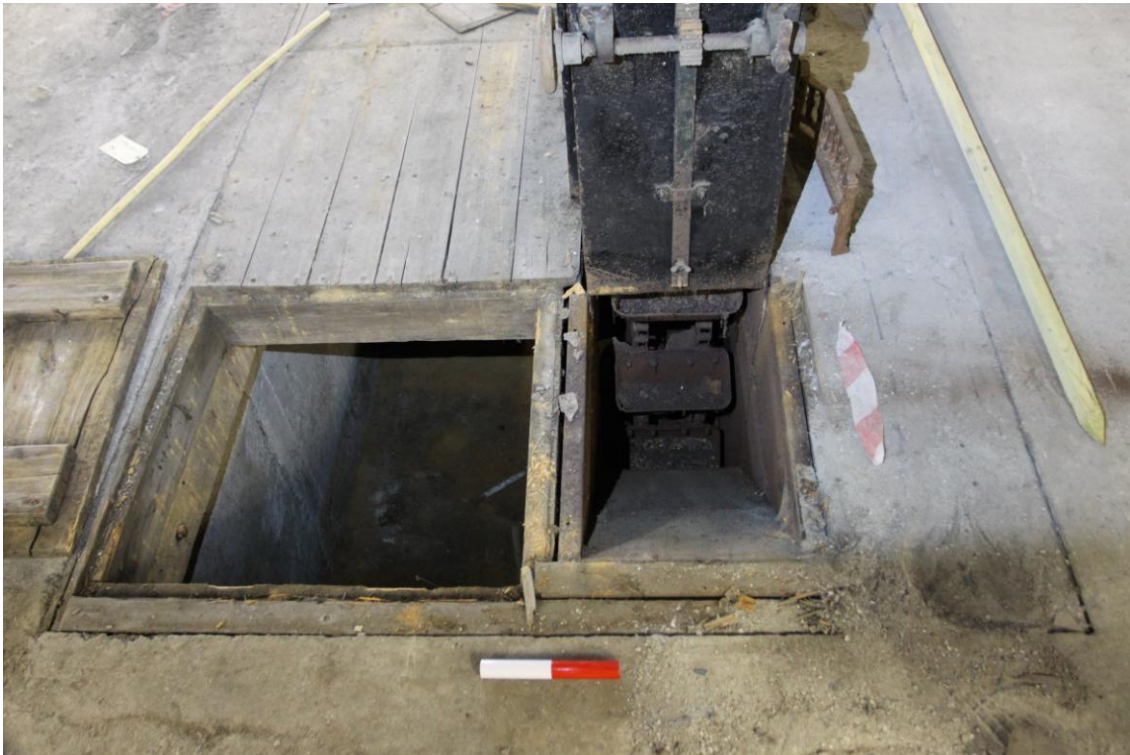
Plate 34: Double Bucket Elevator mechanism and inspection chamber, Ground Floor Level (Photograph 83).
