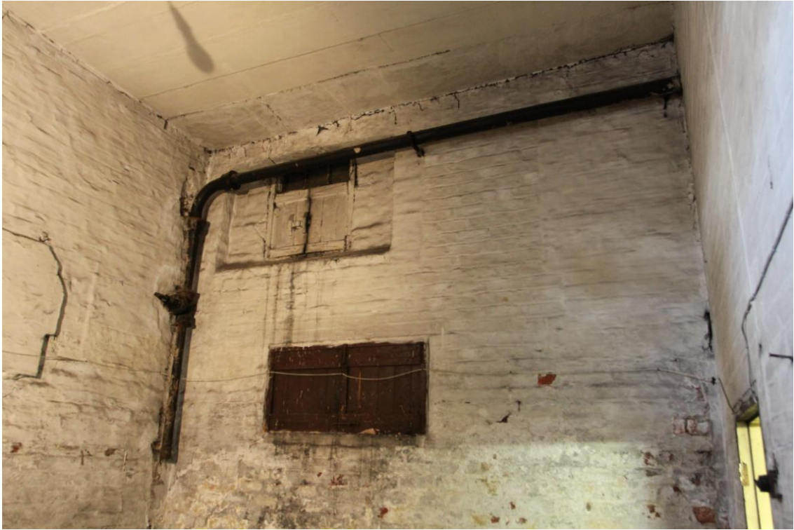
Plate 27: Water Inlet Pipe, West Elevation of Kiln, Ground Floor Level (Photograph 97).
