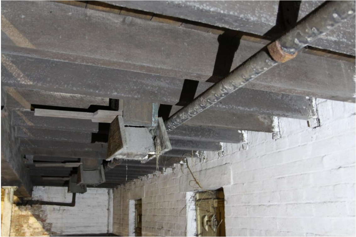
Plate 29: Water Inlet Pipe above Steeping Cistern, punctured with holes and grain chutes (Photograph 159).
