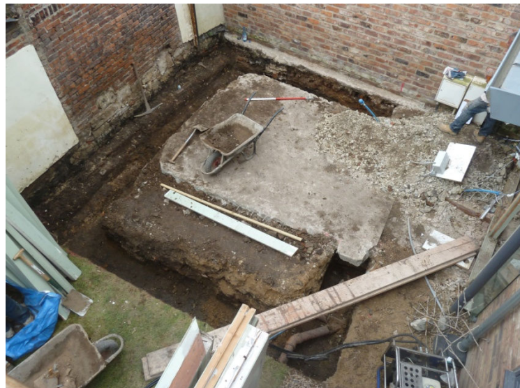
Plate 2. Overall view of site end of day 2 and completion of excavation work looking NW. Scale 1m.
