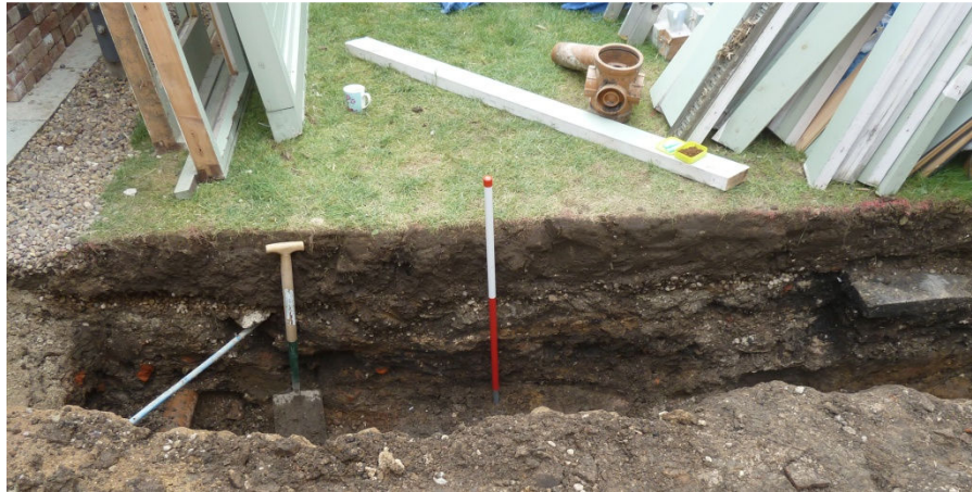
Plate 5. South footing trench, North facing section- East end and middle of section. Scale 1m
