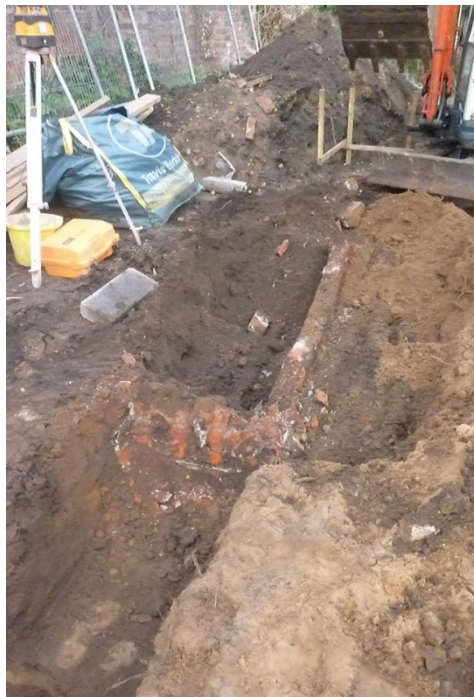
Plate 6. Brick lined feature in North footing trench under removal, looking E. Scale 1m
